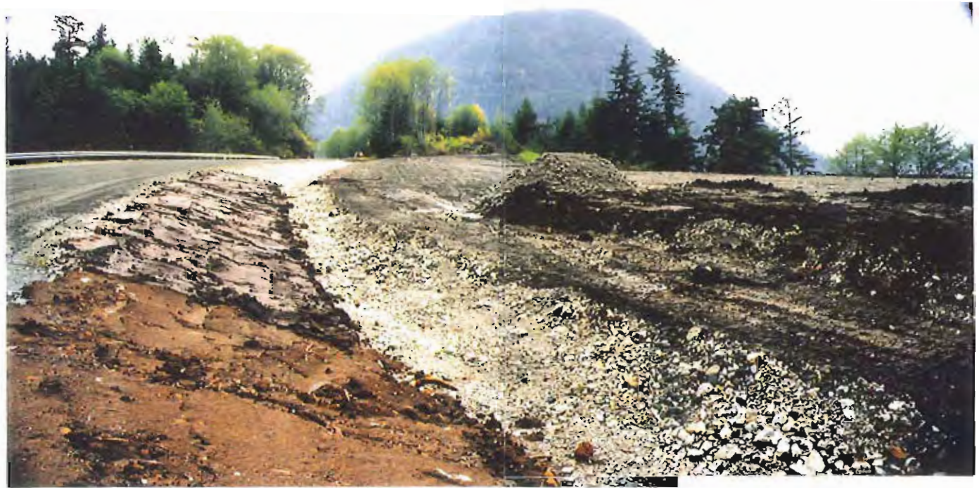
Photo #25: 10/20/99 view looking southeast along the drainage ditchline between the Sawmill Creek Road and the APC/Sitka landfill, showing the initial placement of soil from the roadside to the ditch to insure positive runoff to the membrane-lined ditch.
