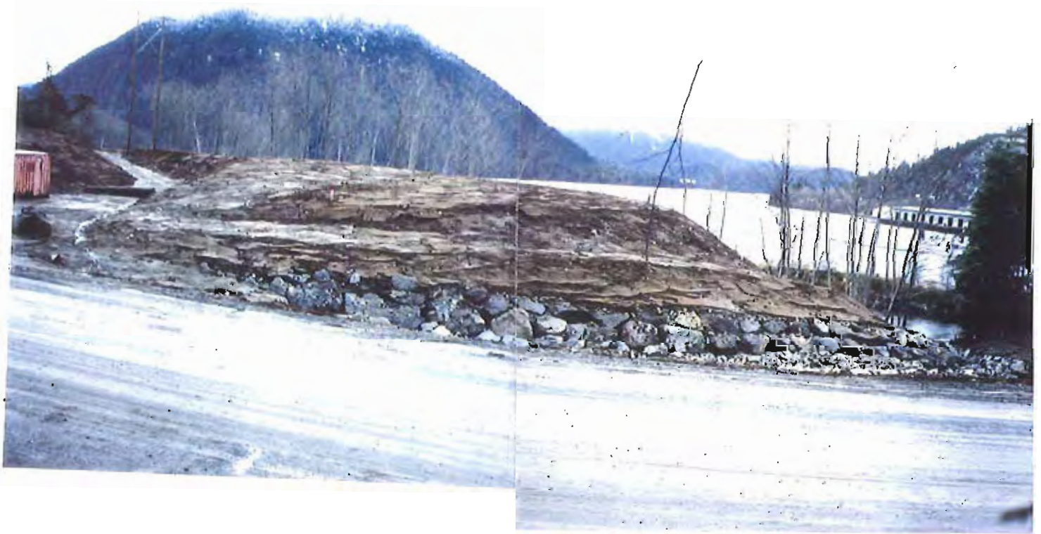
Photo #76: Closer view of the APC/Sitka landfill's northwestern end, showing the completed rockwork along the edge of the open drainage ditch and the final soil cover over the entire area.
