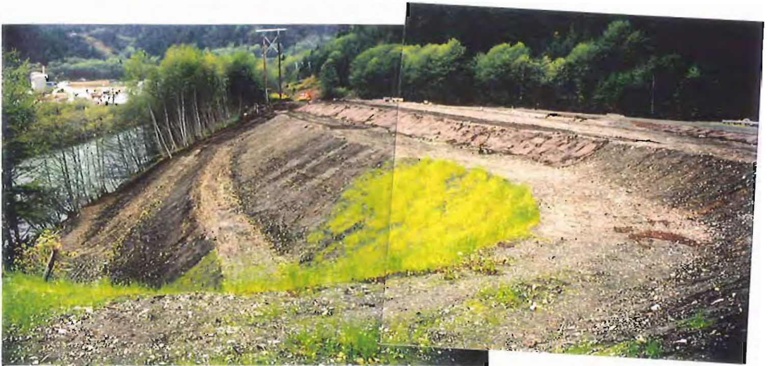
Photo #29: 10/20/99 view looking northwest along the nearly completed embankment area of the APC/Sitka landfill, showing the soil cover that now is in place and ready for grass-seeding.
