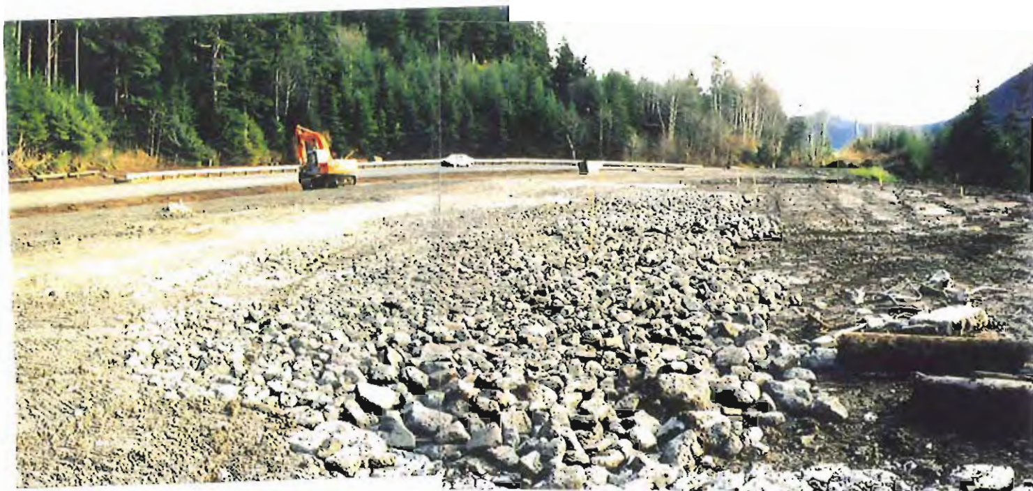
Photo #47: 11/11/99 view looking southeast across the upper surface of the APC/Sitka landfill site, showing the initial 6"-thick layer in the process of being placed. Survey stakes can be seen throughout the area being filled, to make certain that the 18"-thickness will be achieved throughout the area.
