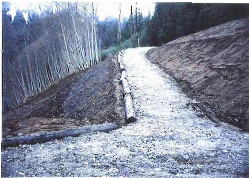
Photo #86: 11/23/99 view looking up the APC/Sitka landfill's embankment roadway, showing the creosoted logs lining the outside edge and the crushed-concrete fill now covering the entire roadway surface. A drainage ditch was created along its inside edge to keep surface water away from the lower embankment slope.
