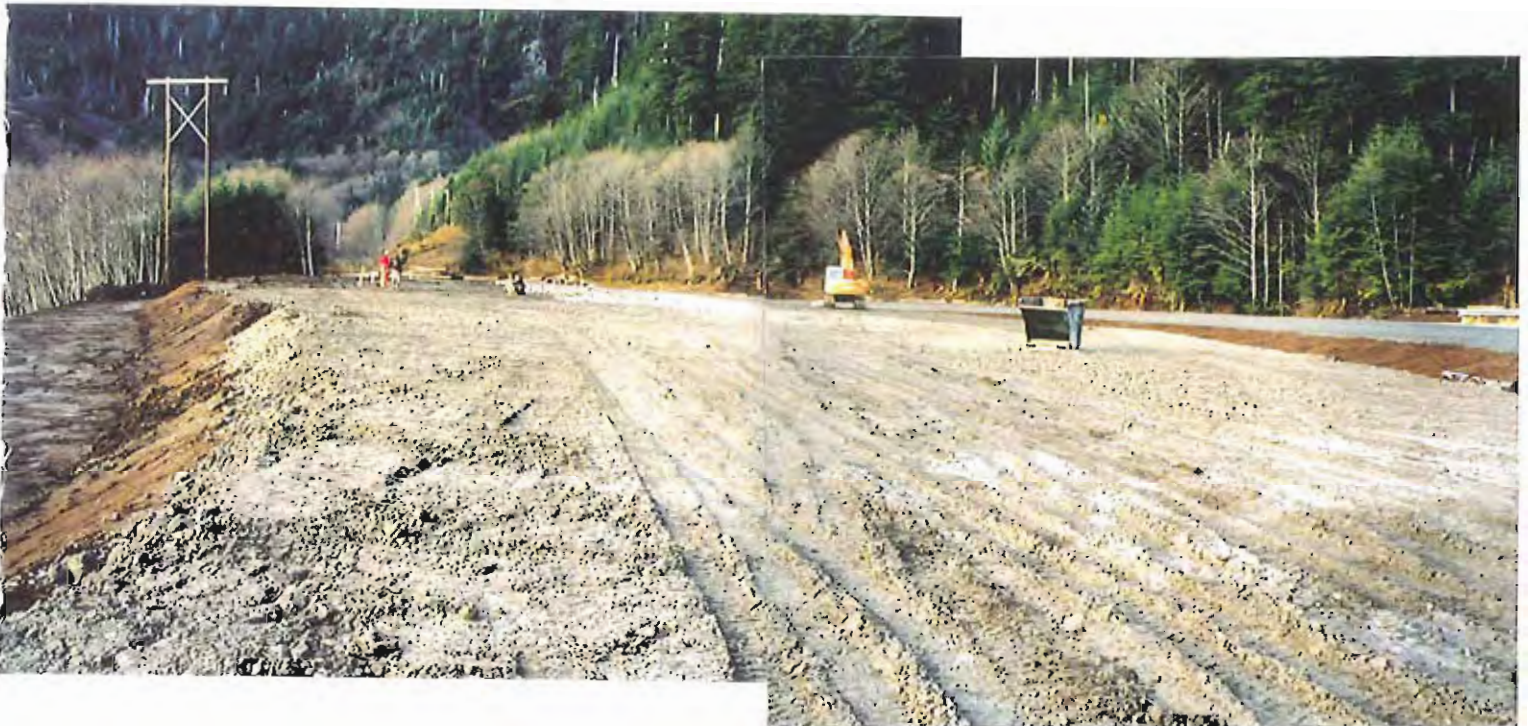
Photo #46: Closer view of the crushed-concrete fill already spread and levelled in preparation for the final 6"-thick covering of soil, 11/11/99. Crushed-concrete fill is continuing to be placed in the far background, where survey stakes are present to guide the final placement of fill.
