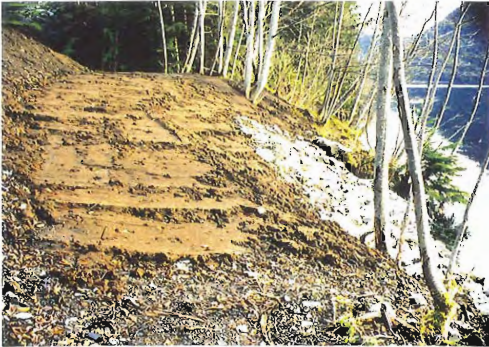
Photo #55: Looking southeast across the top of the tidelands stabilization rockwork at about Sta. 3+00', showing the completed 6"-thick soil layer to extend to the top of the rock and to the undisturbed embankment in the far right of the photo.
