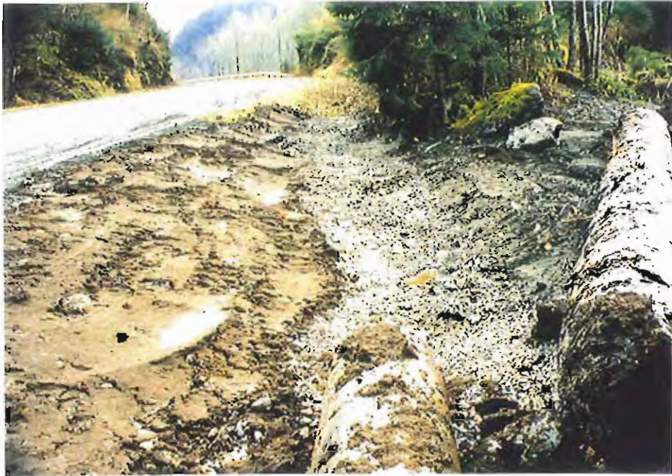
Photo #51: Looking southeast across the end of the Sawmill Creek Roadway's lower ditchline, now completed with its 10'-wide by 30-mil membrane liner completely covered with crushed concrete fill and a soil layer covering the roadside embankment (compare with Photo #8 on page A5).
