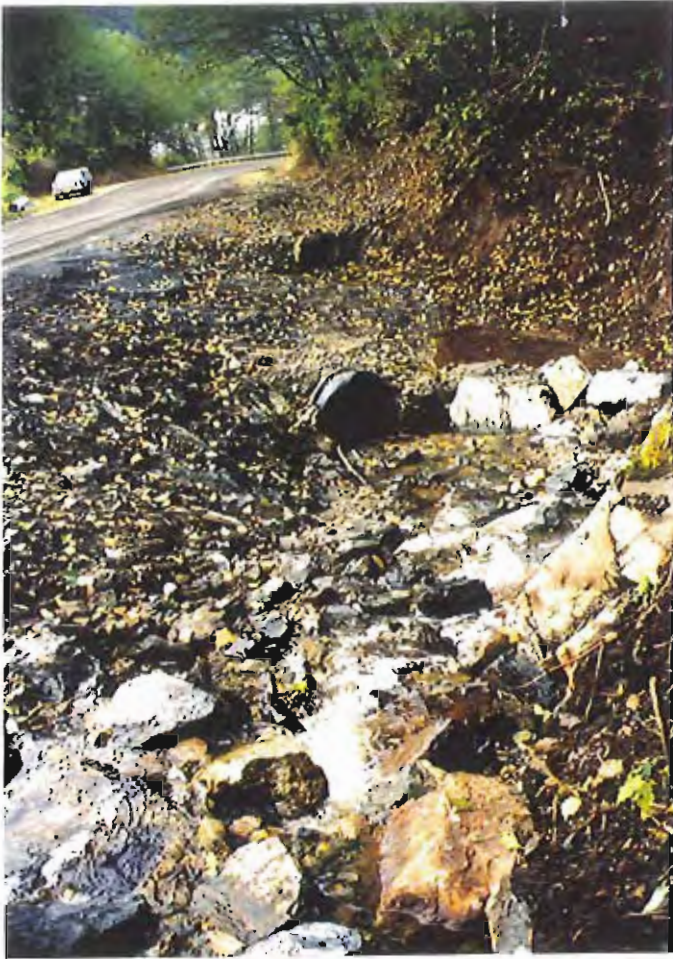
Photo #21: 10/20/99 view of the two 3'-dia culverts now providing positive surface water drainage from along the upland side of Sawmill Creek Road. The new culvert in the foreground is about 4' lower than the old culvert.
