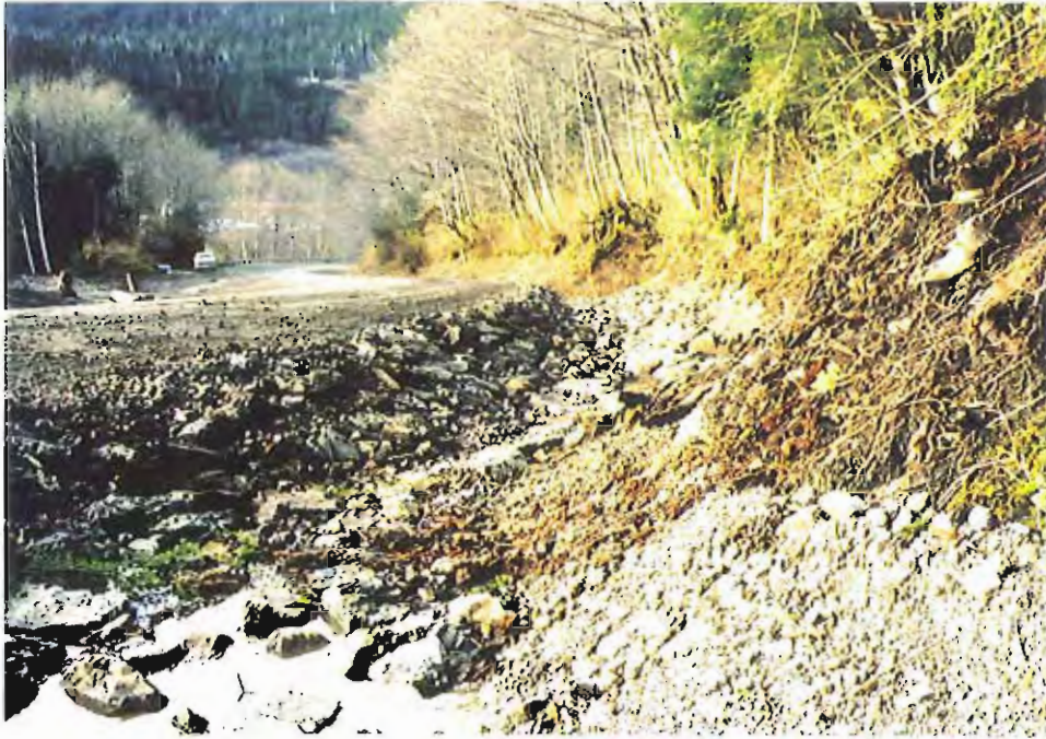
Photo #9: Looking down the Sawmill Creek Road's upslope surface water drainage ditch from about Sta. 3+80', showing the large rock placed in the ditchline to prevent erosion of the protective rock cover over the underlying 30-mil membrane liner, 11/11/99.
