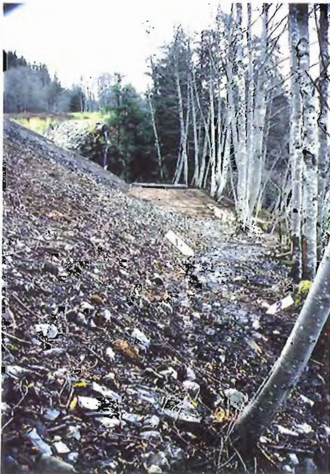
Photo #88: Looking southeast along the embankment toe of the APC/Sitka landfill from about Sta. 4+00', showing two very small water seepage areas (see next 3 photos)
