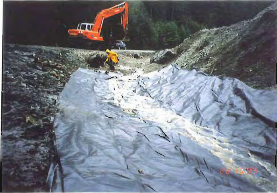
Photo #15: Earlier 10/28/99 view of placing the 20'-wide by 30-mil membrane liner in the surface water drainage ditch just below the Sawmill Creek Road's culvert at the APC/Sitka landfill's northwestern end (compare with Photo #14).
