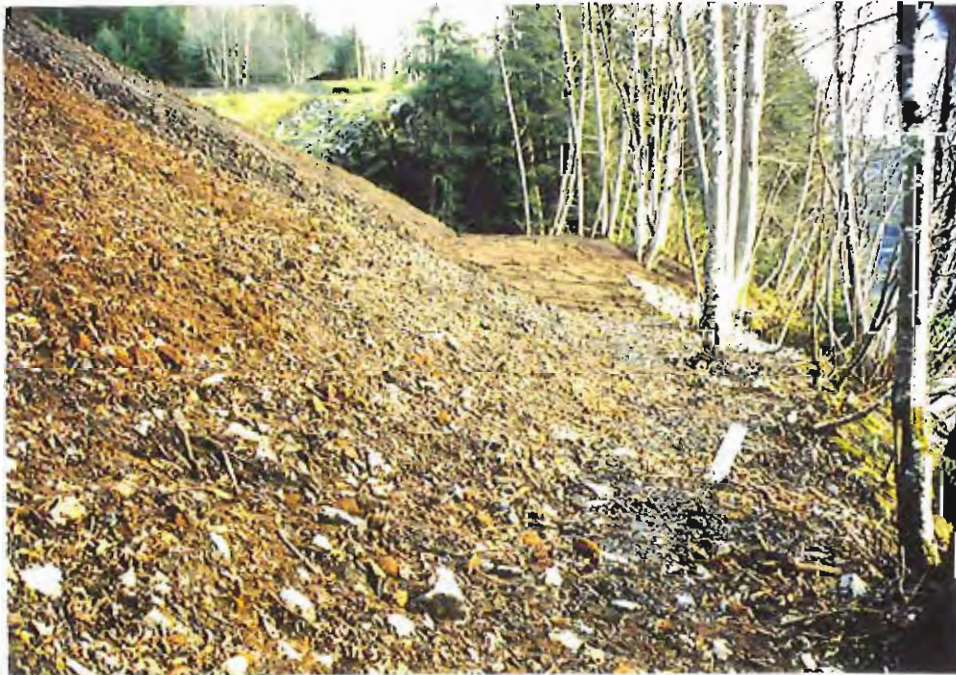
Photo #58: Closer 11/11/99 view of a damp soil area at about Sta. 3+50' along the APC/Sitka landfill's embankment toe, where a very small unmeasurable water seepage appears to be present.
