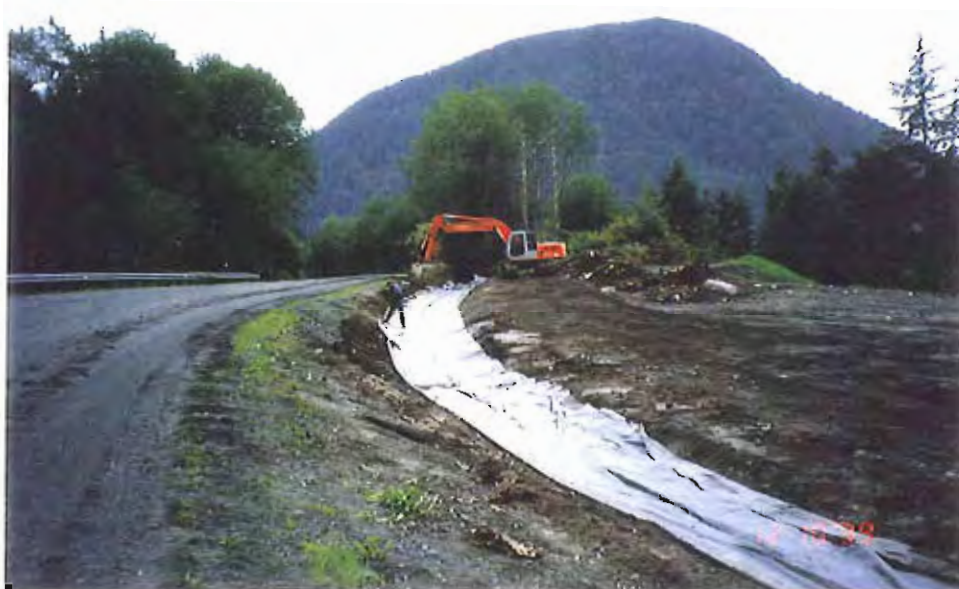
Photo #18: Earlier 10/12/99 view of the 10'-wide by 30-mil membrane liner being laid to the end of the downslope surface water ditch along the Sawmill Creek Road, near the southeastern end of the APC/Sitka landfill site (compare with Photo #3).
