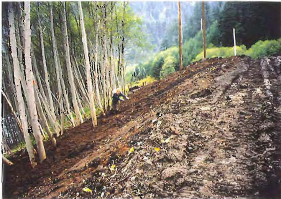
Photo #32: Hand-raking and smoothing out of the embankment soil along about Sta. 3+50', 10/20/99.
