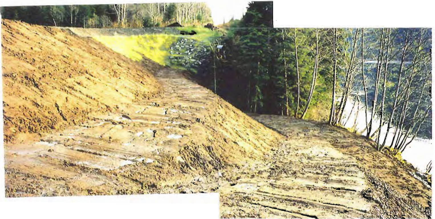
Photo #54: 11/11/99 view looking southeast across the mid-&-lower levels of the APC/Sitka landfill's embankment, showing the entire area to be covered with its final 6"-thick layer of soil.
