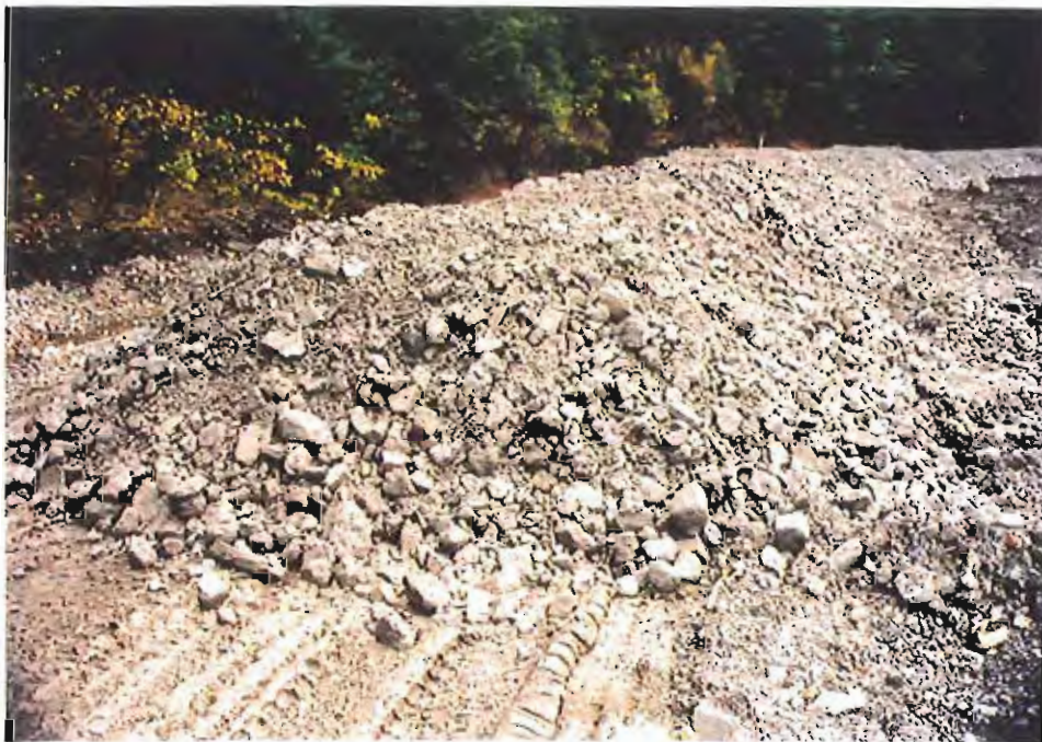
Photo #28: Close-up view of the crushed rock being loaded out for placement over the APC/Sitka landfill's northeastern area, showing its clean and porous appearance.
