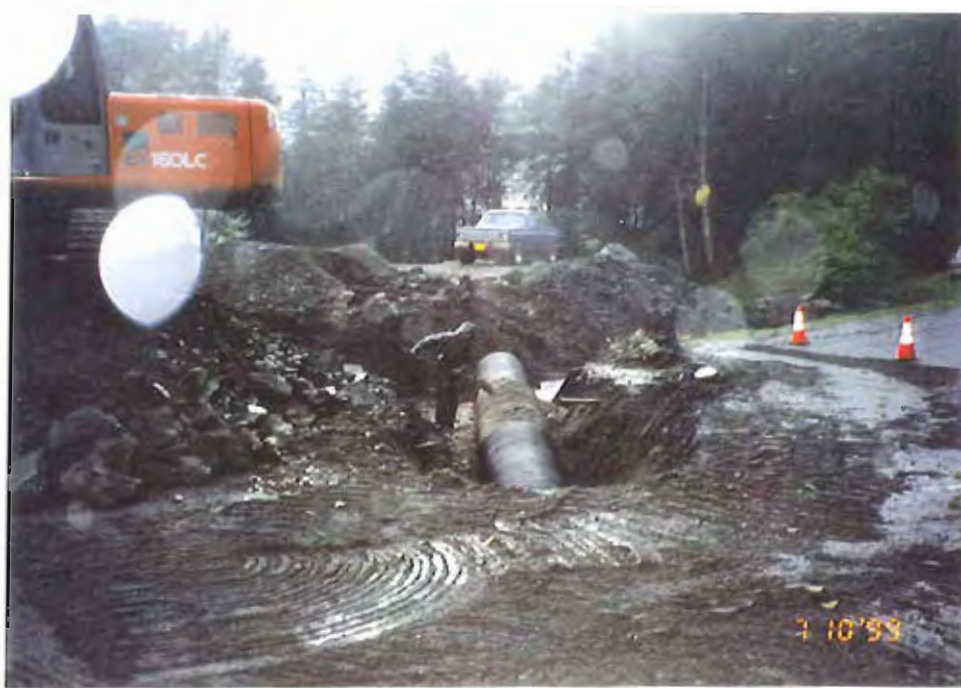
Photo #1: 10/7/99 view of the initial section of new 3'-dia. culvert being installed across the Sawmill Creek Roadway near Sta. 6+50' of the APC/Sitka landfill site.
