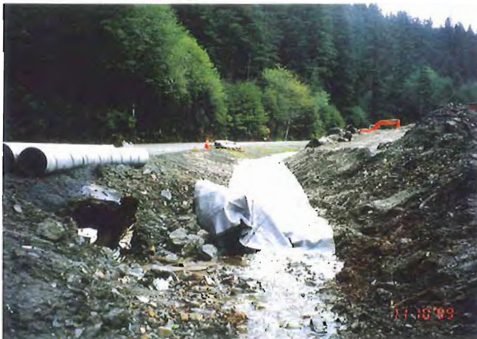
Photo #4: 10/11/99 view of the Sawmill Creek Road's downslope drainage ditch, just after the 10'-wide 30-mil membrane material had been rolled out.
