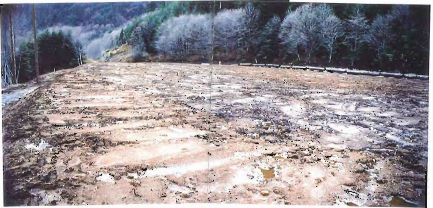
Photo #81: Looking northwest across the main top area of the APC/Sitka landfill site on 11/23/99, showing its smoothed-out surface and the fill stakes placed to confirm the needed depth of the underlying 18"-thick crushed concrete rock and the top 6"-thick soil cover (compare with photos on page A25).
