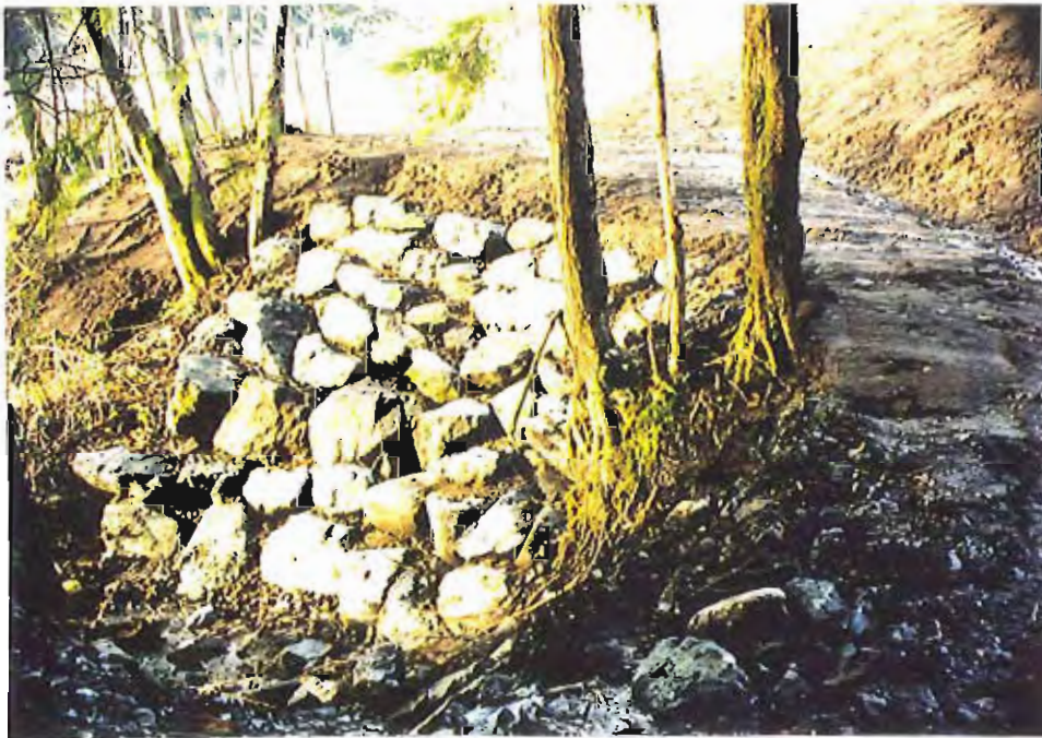
Photo #56: 11/11/99 view of the completed stabilization rockwork along the bottom toe of the APC/Sitka landfill embankment at about Sta. 1+30'. Also shown is the completed 6"-thick layer of soil over the upper pathway and along the lower embankment to the left side of the rockwork.
