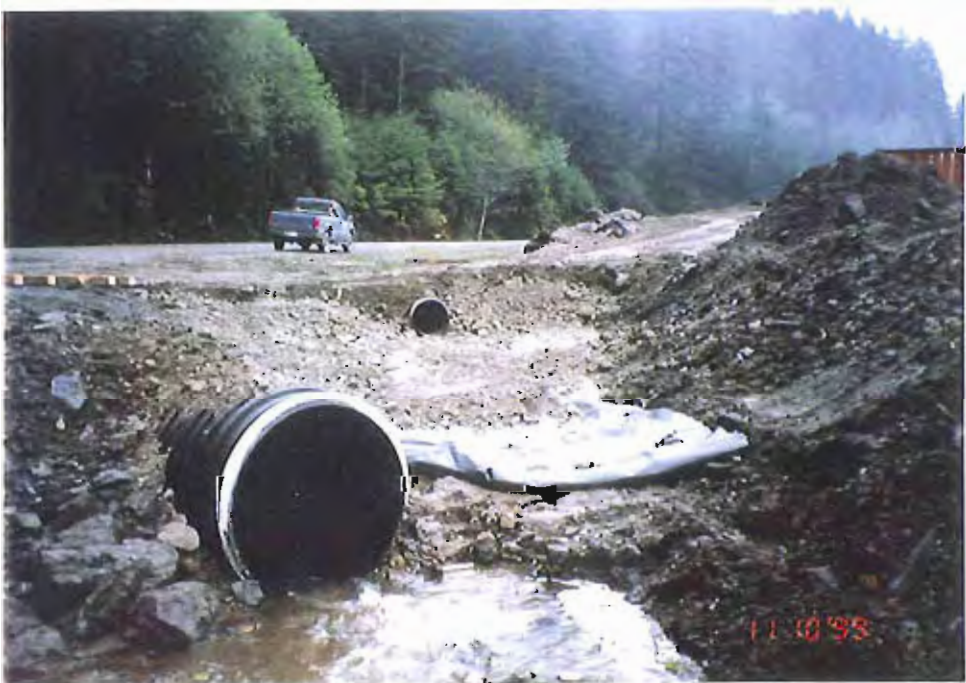
Photo #6: View of the downslope drainage ditch between the Sawmill Creek Roadway and the APC/Sitka landfill on 10/11/99, showing the 6" layer of crushed concrete and the 30-mil membrane below the now-installed 18"-dia culvert under the APC/Sitka landfill's access road.
