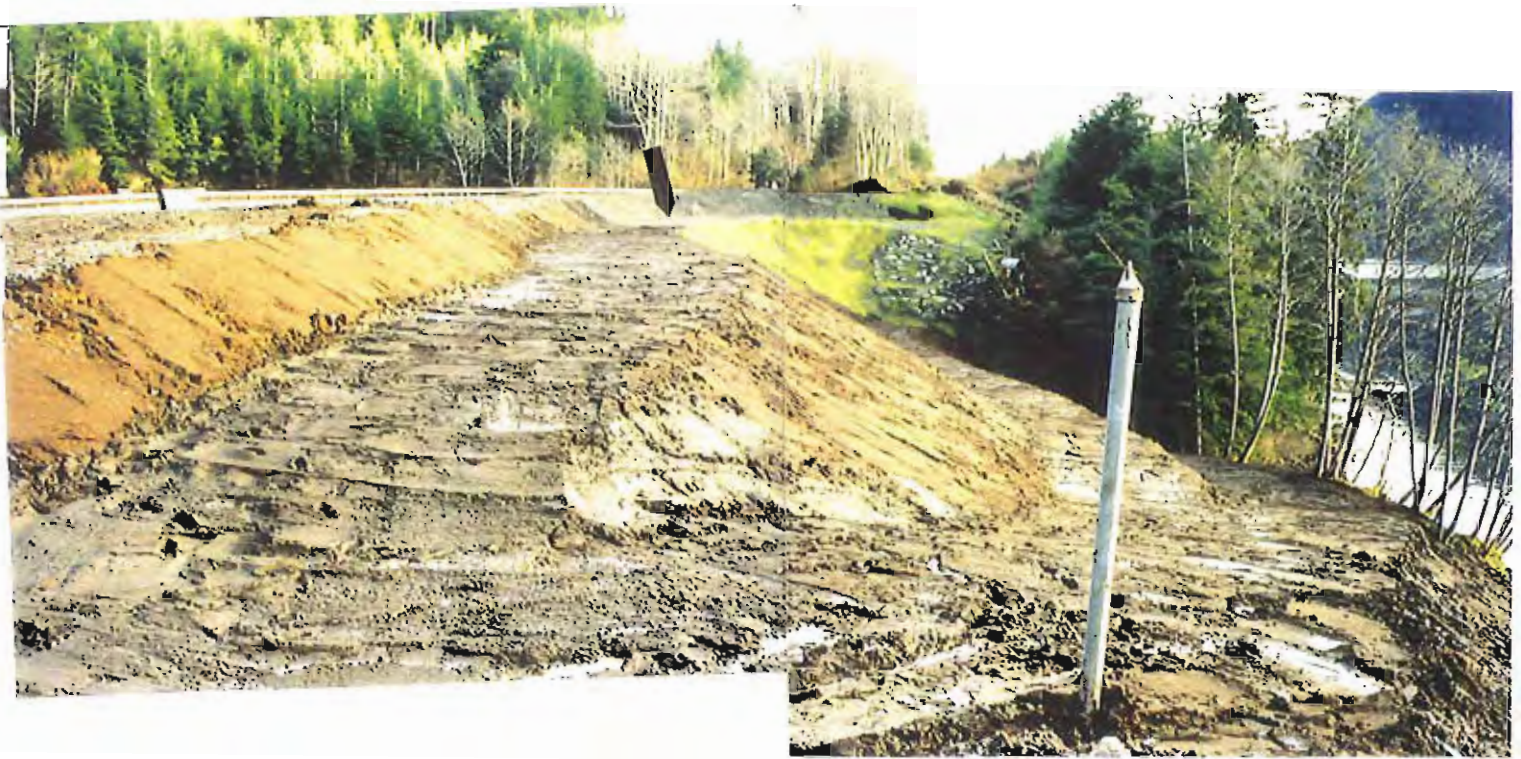
Photo #53: Looking southeast across the upper embankment of the APC/Sitka landfill on 11/11/99, showing it to be completely covered with a 6"-thick layer of soil. The only area still remaining to be covered is just beyond the arrow.
