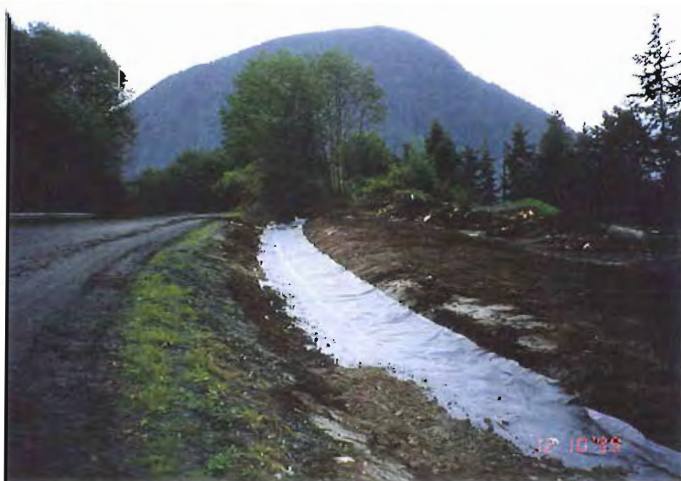
Photo #8: 10/12/99 placement of the 30-mil membrane along the upper end of the of the surface water drainage ditch between the APC/Sitka landfill and the Sawmill Creek Road, showing the careful securing of the membrane's edge within the adjacent roadside soil.
