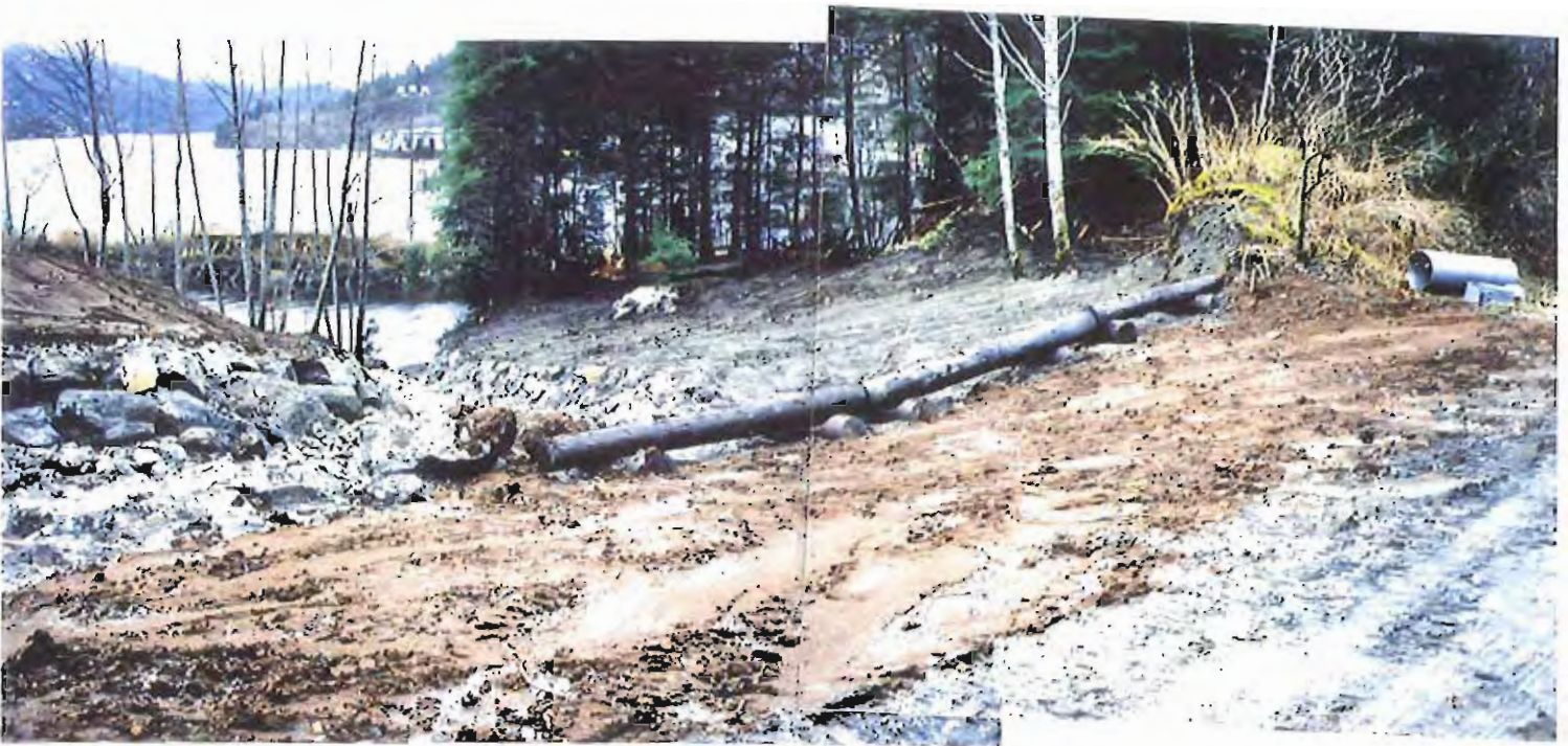
Photo #77: 11/23/99 view looking down the open ditch around the northwestern end of the APC/Sitka landfill, showing the rocked open drainage ditch and the landscaped area on its far side where the site meets the undisturbed forested area.
