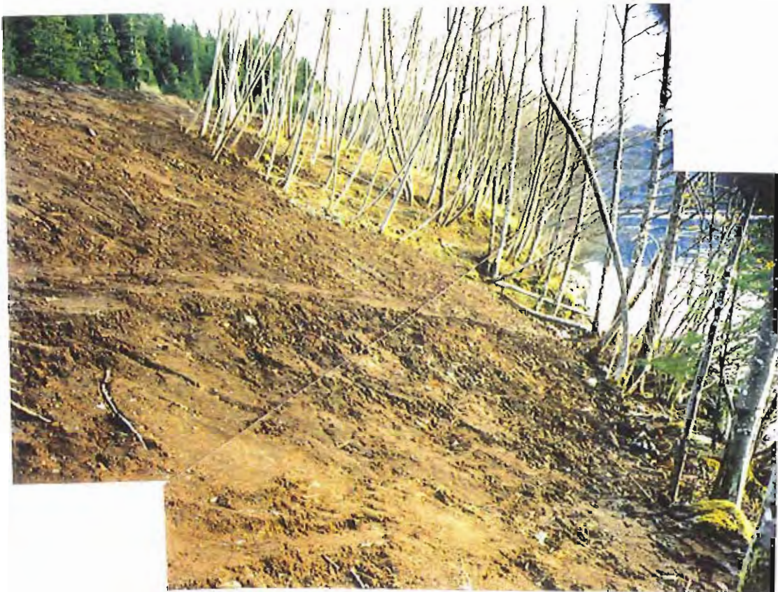
Photo #70: Looking across the lower portion of the APC/Sitka landfill's northwestern embankment area (photo taken from the embankment edge near the drainage ditch), showing the completed 6"-thick soil layer across the entire area and that has been merged into the undisturbed soil along its edge.
