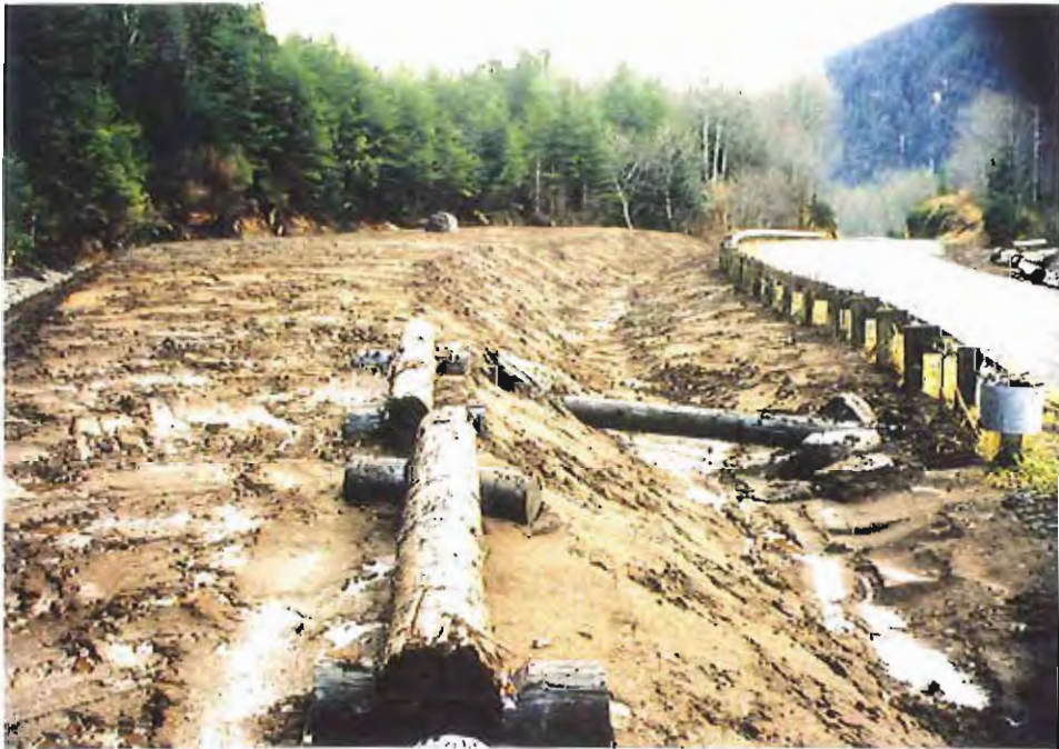
Photo #62: 11/11/99 looking up the completed roadside ditchline between the Sawmill Creek Roadway and the APC/Sitka landfill's northeastern fill area, and the area's now-completed layer of 6"-thick soil.
