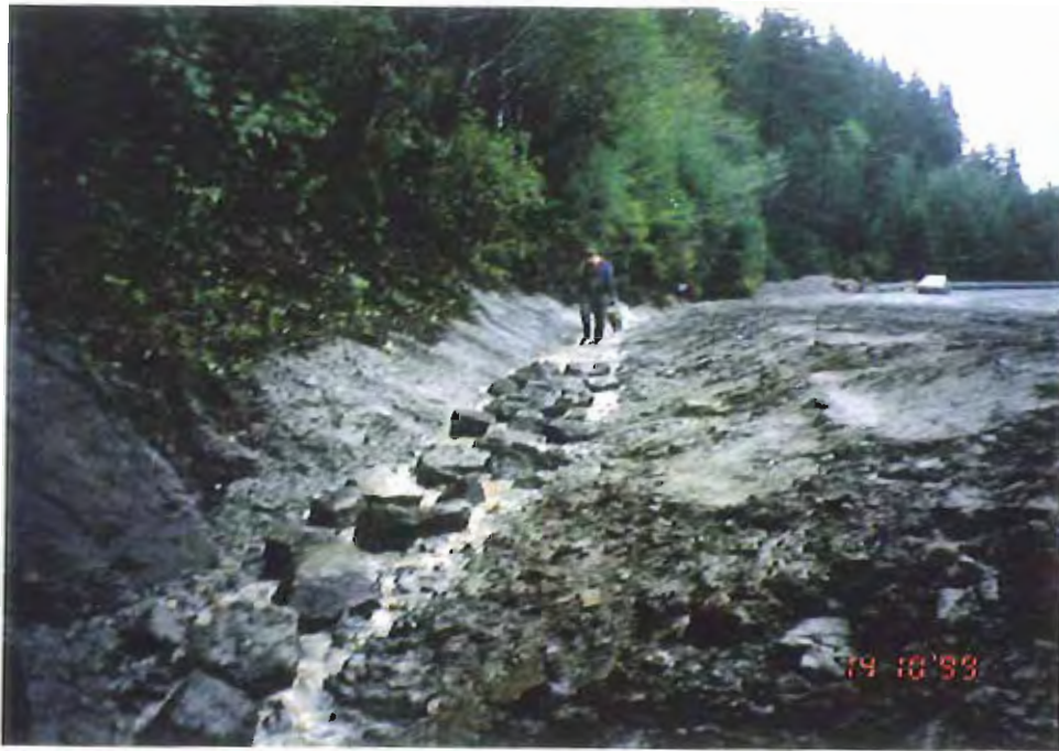
Photo #17: 10/14/99 placement of large rock to protect against erosion in the nearly completed drainage ditch along the Sawmill Creek Road's upland side at the APC/Sitka landfill site.
