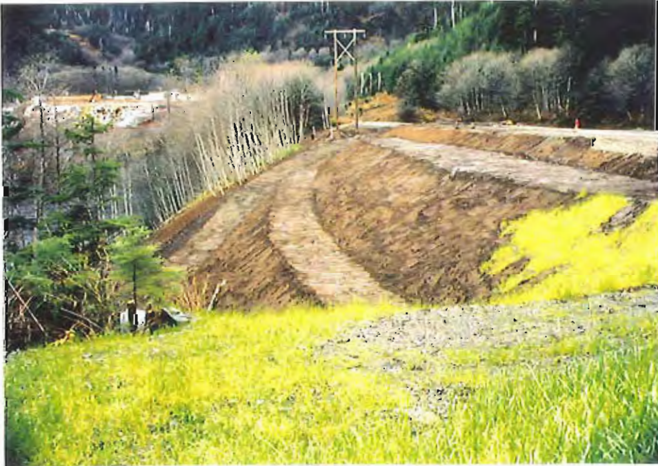
Photo #52: Looking northwest across much of the APC/Sitka landfill's main embankment area, showing the final 6"-thick layer of soil to be in place except for the far right-hand edge of the photo.
