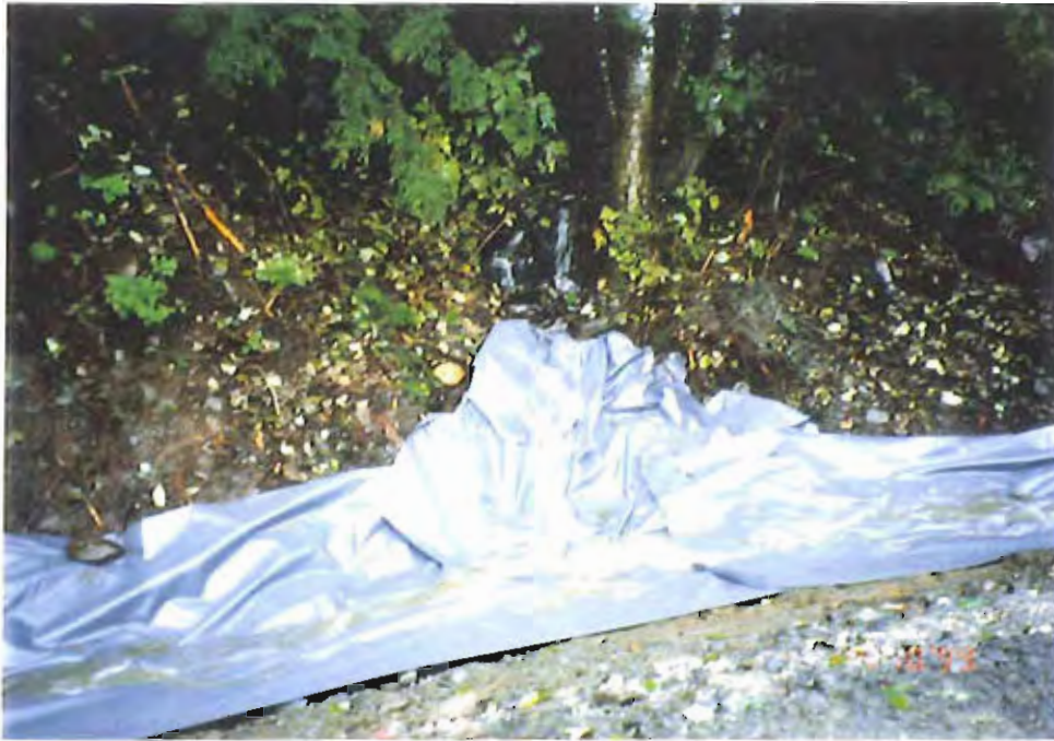
Photo #15: Extension of the 30-mil membrane liner to catch the runoff from a small upland creek at about Sta. 4+70' of the APC/Sitka landfill site, along the upland side of Sawmill Creek Road, 10/14/99.
