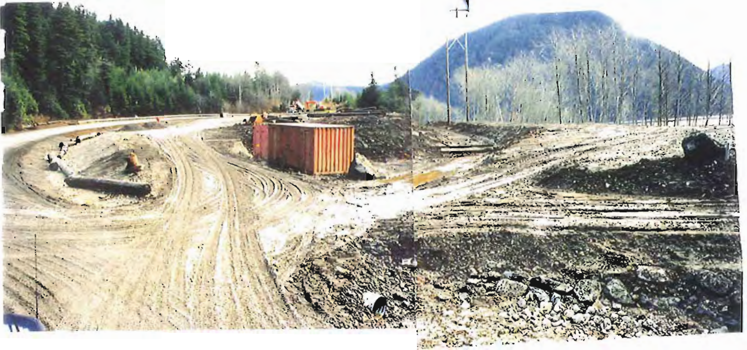
Photo #37: 11/11/99 view of the APC/Sitka landfill's entrance area, showing the completed roadside ditch and logs in the ditch in preparation for final placement along the top outside top of the ditch once the surfacing fill and soil are completed.
