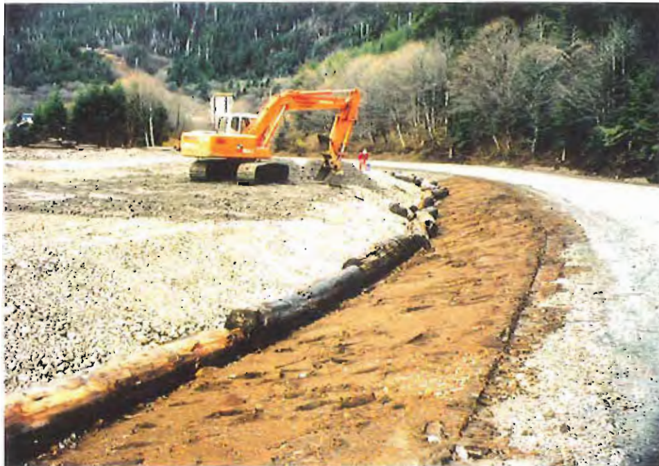
Photo #44: Closer view of the backhoe spreading the crushed concrete fill in thin layers along the APC/Sitka landfill's roadside ditch, 11/11/99. A laborer can be seen watching out for and picking up any remaining pieces of metal that might be seen in the fill material.
