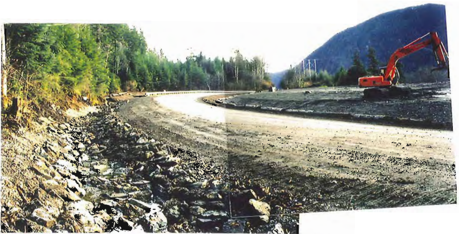
Photo #59: Looking south across the Sawmill Creek Road from about Sta. 3+50', showing the completed upslope ditchline including its armor rock on the right side of the photo, 11/11/99.
