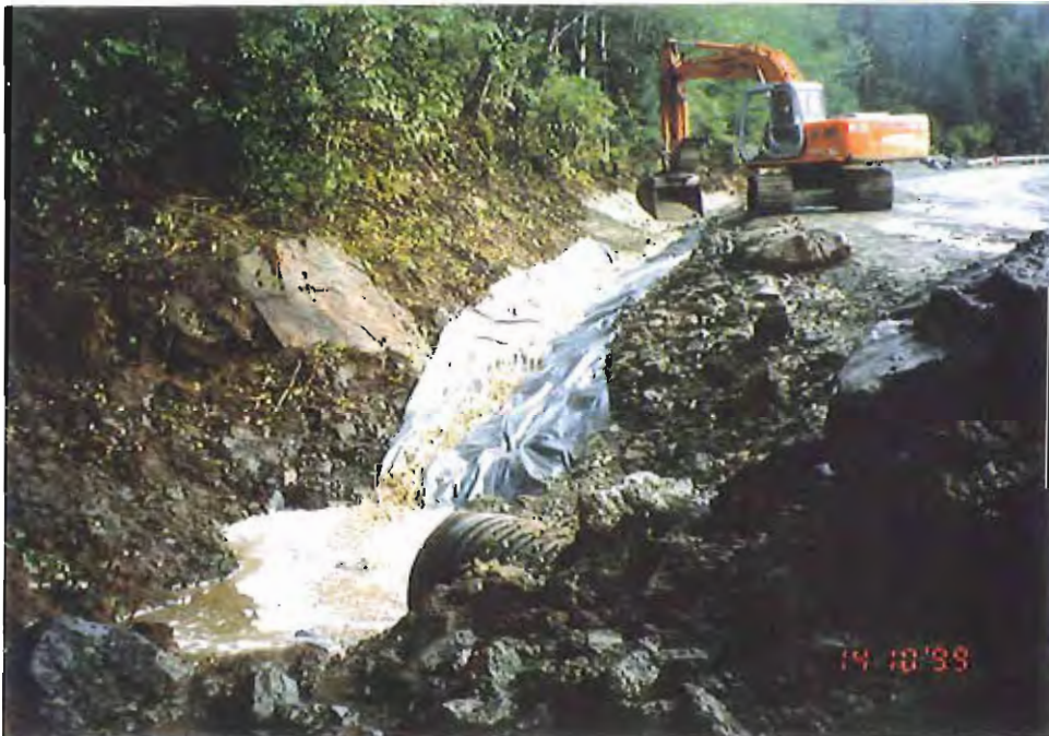
Photo #16: Looking across the inlet of the new 3'-dia. culvert now carrying all of the upland surface water drainage across the Sawmill Creek Road at about Sta. 6+40' of the APC/Sitka landfill site, 10/14/99.
