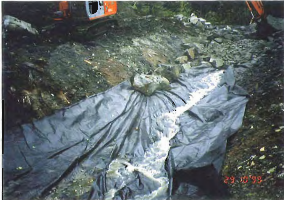
Photo #35: 10/29/99 view of the APC/Sitka landfill's northwestern ditch, showing the protective rock layer being placed over the 20'-wide by 30-mil membrane liner. Large rock is placed along and on the upper edges of the liner, with a 1'-thick layer of smaller rock placed across the inner surface of the liner.
