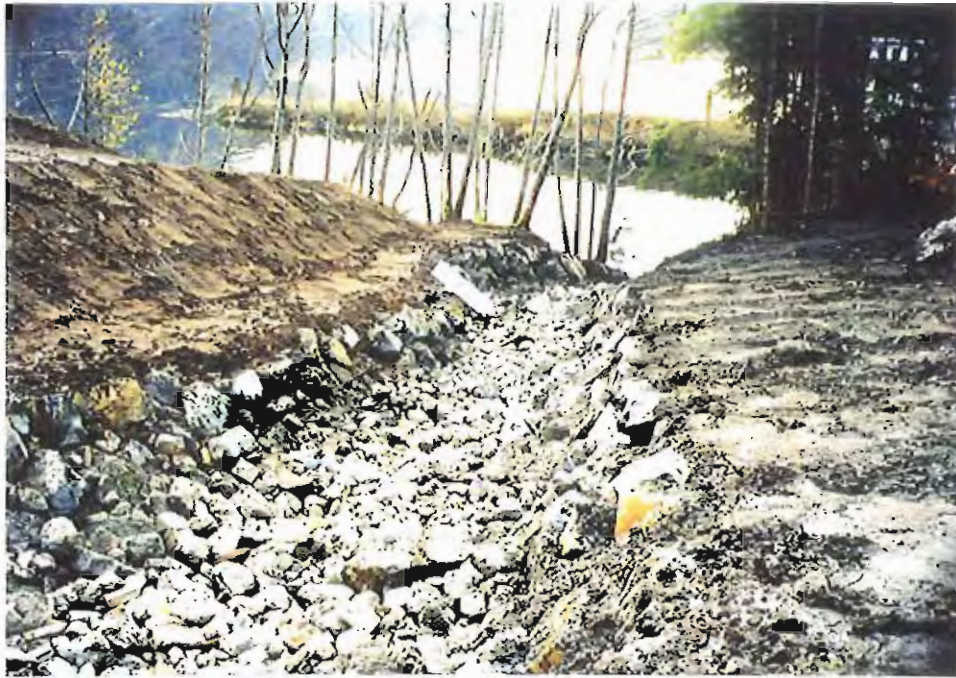
Photo #41: 11/11/99 view across the bottom area of the APC/Sitka landfill's northwestern drainage ditch. The 20'-wide by 30-mil membrane liner now is completely covered with 6"-8" rock to protect against erosion. The arrow shows where the membrane liner ends, after which hard rock makes up the bottom of the ditch.
