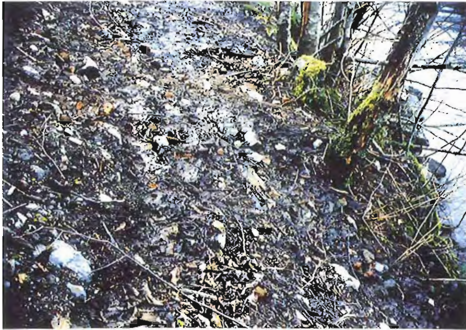
Photo #91: Closer 11/23/99 view of the very small water seepage #2 along the APC/Sitka landfill's embankment toe at about Sta. 3+60' (see Photos #88-#89 for location).
