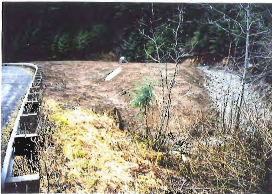
Photo #4: Looking across the end of the upper end of the APC/Sitka landfill's northeastern disposal area, showing the new roadside drainage ditch along Sawmill Creek Road (see arrow).
