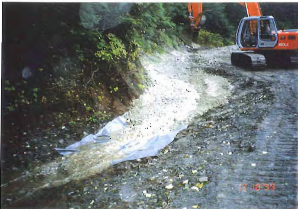
Photo #12: Continuing work on the APC/Sitka landfill's upslope ditch along the northeastern area, showing the 30-mil membrane and 6" of overlying crushed concrete cover, 10/13/99. Note the substantial water runoff.
