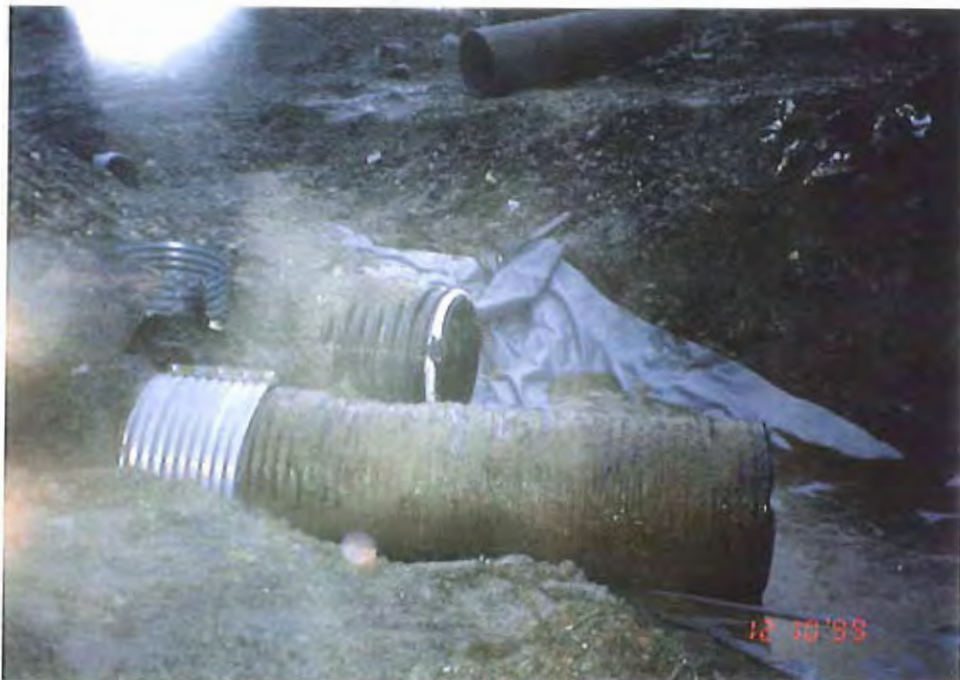
Photo #9: 10/12/99 view of the culvert extension and band placed on the end of the original 3'-dia culvert, to extend it further away from the edge of the Sawmill Creek Roadway.
