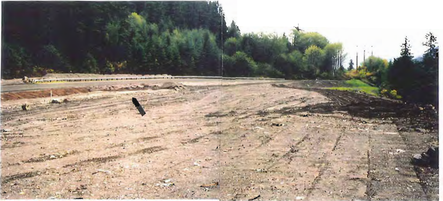
Photo #23: 10/20/99 view looking southeast across the upper surface of the APC/Sitka landfill surface from about Sta. 4+00', showing the well-compacted top surface of the fill. Also shown is the 1.5' lift of new crushed-concrete rock (see arrow) that eventually will cover the entire surface of the landfill.
