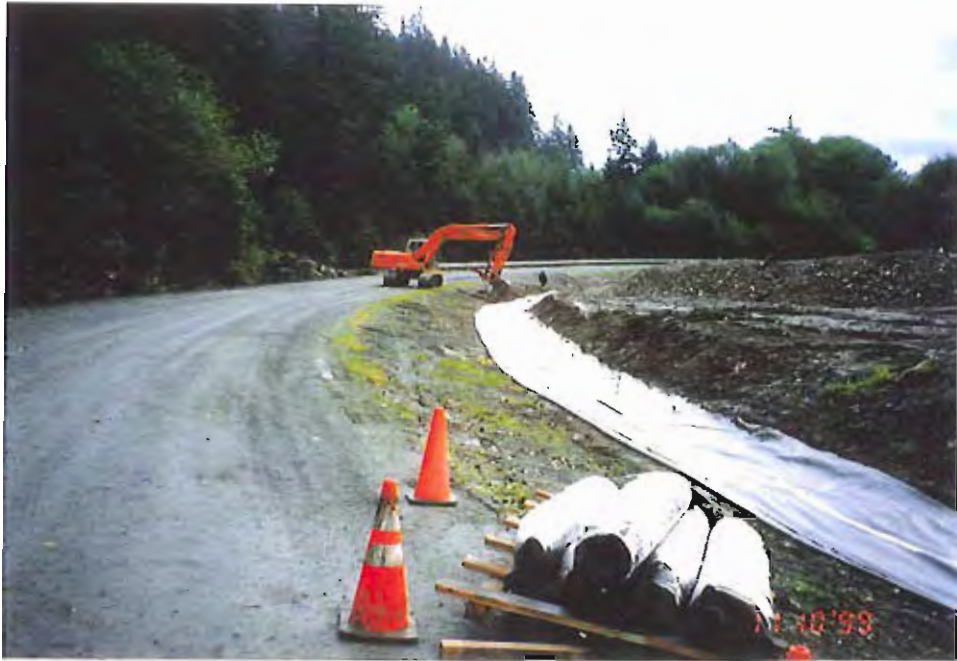
Photo #7: Continued laying and securing of the 10 3 -wide 30-mil membrane along the downslope water drainage ditch between the Sawmill Creek Road and the APC-Sitka landfill on 10/11/99.
