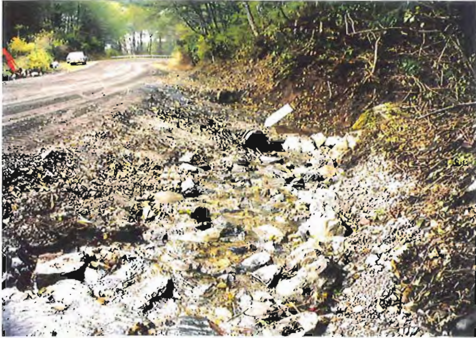
Photo #11: 11/11/99 view of the 3'-dia. culvert inlets going diagonally across Sawmill Creek road near the northwestern end of the APC/Sitka landfill. The new culvert (see arrow) takes all of the water flow, and the old culvert in the background is unlikely to experience any water except during extreme-flood conditions.
