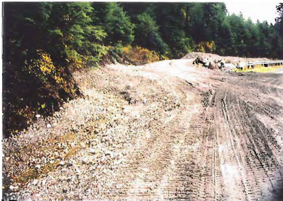
Photo #18: 10/20/99 view at about Sta. 3+20' of the APC/Sitka landfill project site, where the upland drainage ditch flows from the northeastern fill area above the Sawmill Creek Road. Note the considerable volume of water flowing in the ditch, where previously no water had ever flowed.
