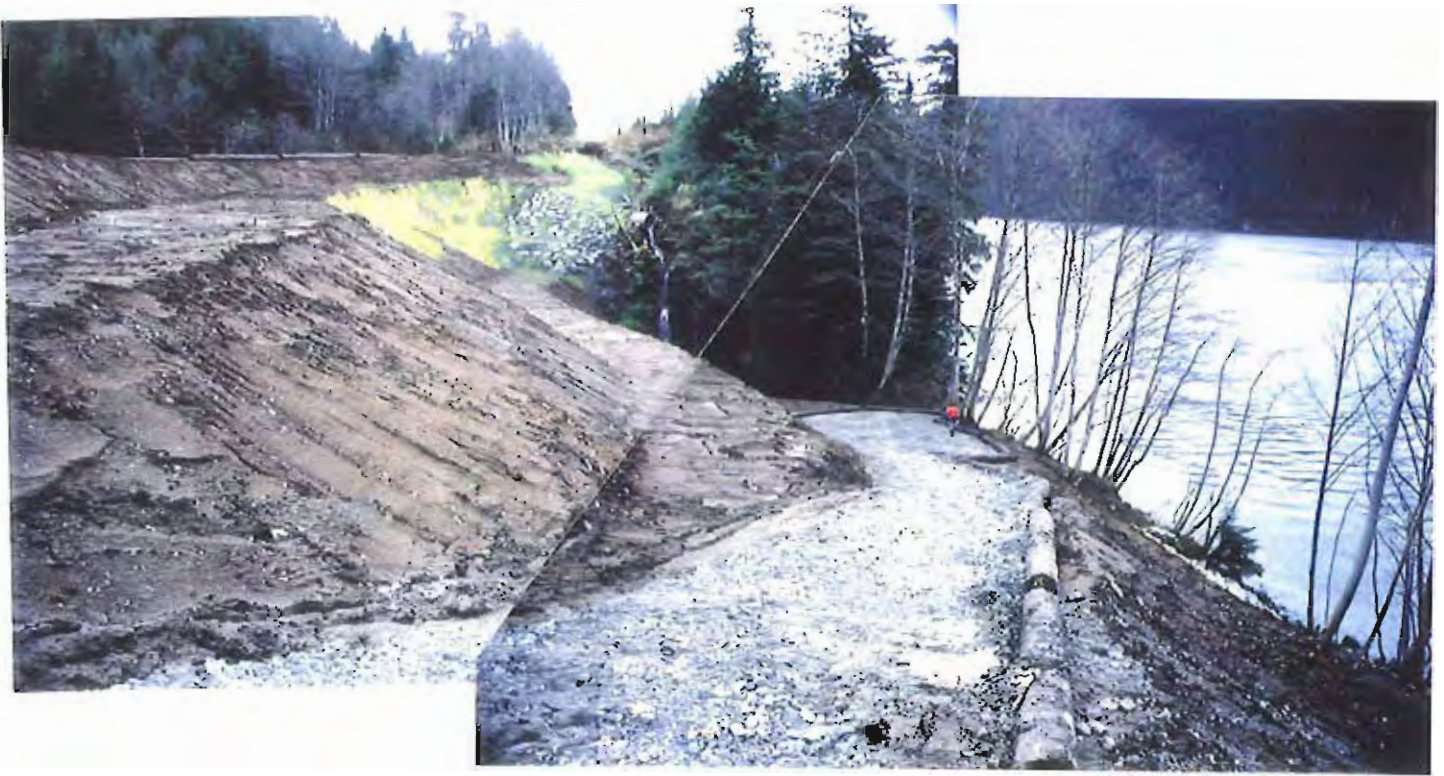
Photo #85: 11/23/99 view looking southeast along the APC/Sitka landfill's terraced embankment slopes, showing the completed soil layer and the access road with its lower turn-around area now surfaced with crushed-concrete fill and lined with creosoted logs.
