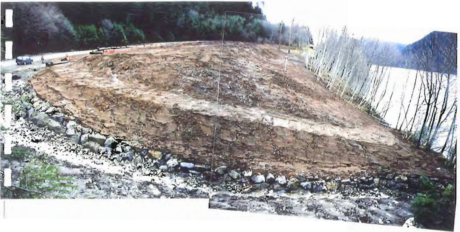
Photo #95: 11/23/99 view looking across the northwestern end of the APC/Sitka landfill, showing the final 6"-thick soil cover over the entire fill surface and the rock lining the surface water drainage ditch embankment (compare with Photo #38, page A20).
