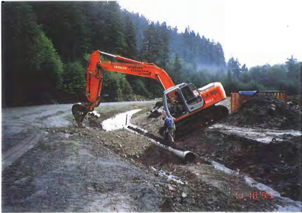
Photo #5: 10/11/99 placement of the 18"-dia culvert at the entrance to the APC/Sitka landfill site, showing the 6" of crushed-concrete fill placed between the membrane and the culvert.
