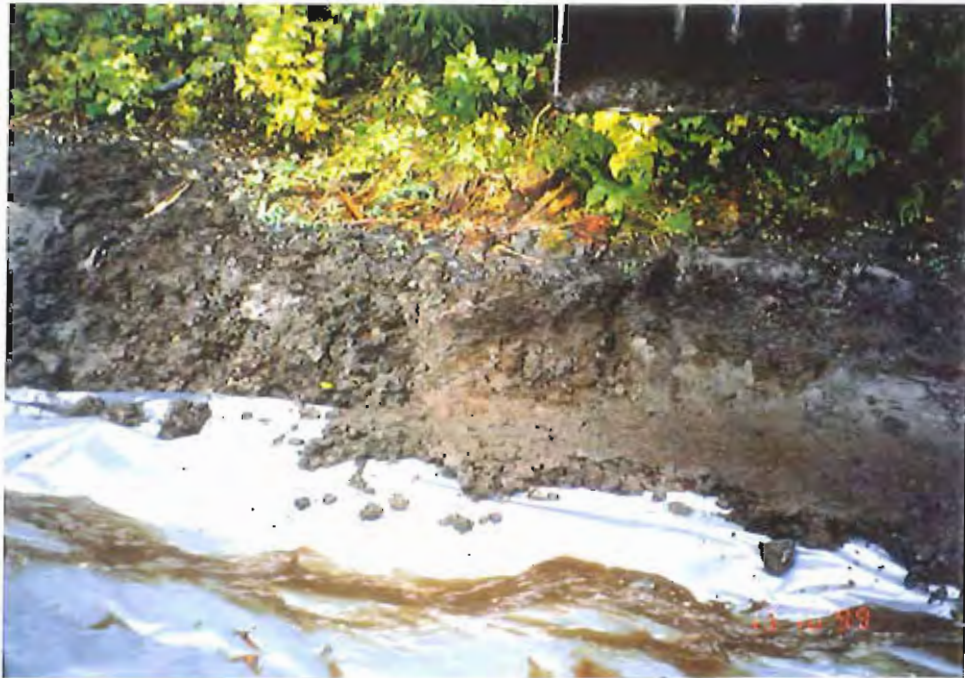
Photo #11: 10/12/99 close-up view of the 30-mil membrane edge being secured into the soil embankment, to assure positive drainage of all upslope water from the APC/Sitka landfill's northeastern area.
