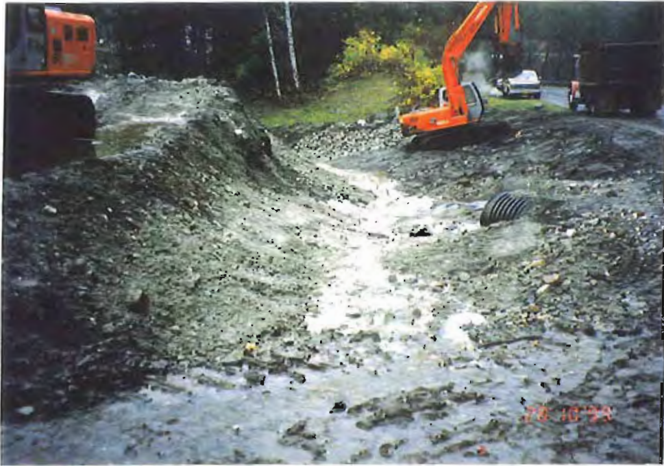
Photo #33: 10/28/99 view of the drainage ditch just below the culvert, with the subbase gravels prepared for placing the 30-mil membrane liner. Note that the ditchline is moved further away from the roadside, and now goes directly over where the large tree stump shown in Photo #22 (see page A12) had been located.
