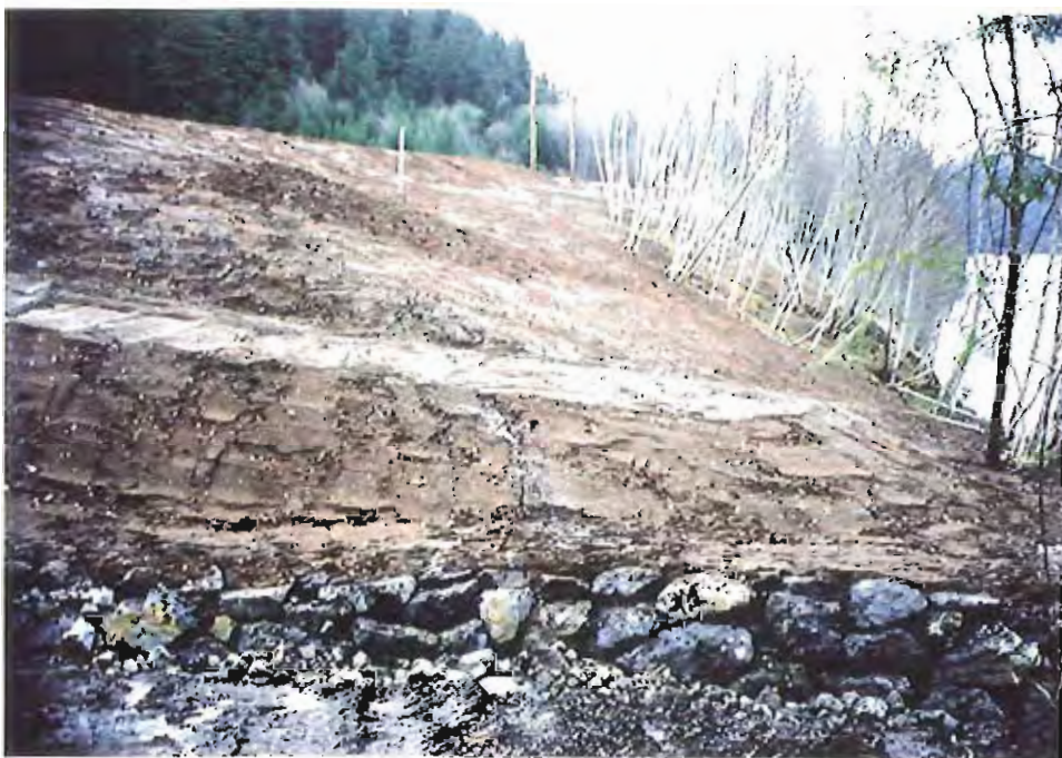
Photo #92: 11/23/99 view looking across the APC/Sitka landfill's northwestern lower embankment slopes, showing the protective rock along the surface water drainage ditch and the completed 6"-soil layer covering all slopes. Arrow points to the water sampling location #1, shown on the next photo).
