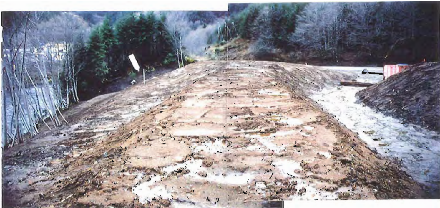
Photo #79: 11/23/99 view looking across the top area of the APC/Sitka landfill's northwestern end, showing the completed 6"-thick soil cover. Arrow points to the cornerpost still remaining as a reference point from the asbestos cyclone fencing taken down at the start of the post-closure improvements project. The post will be cut down once the as-built survey is completed.
