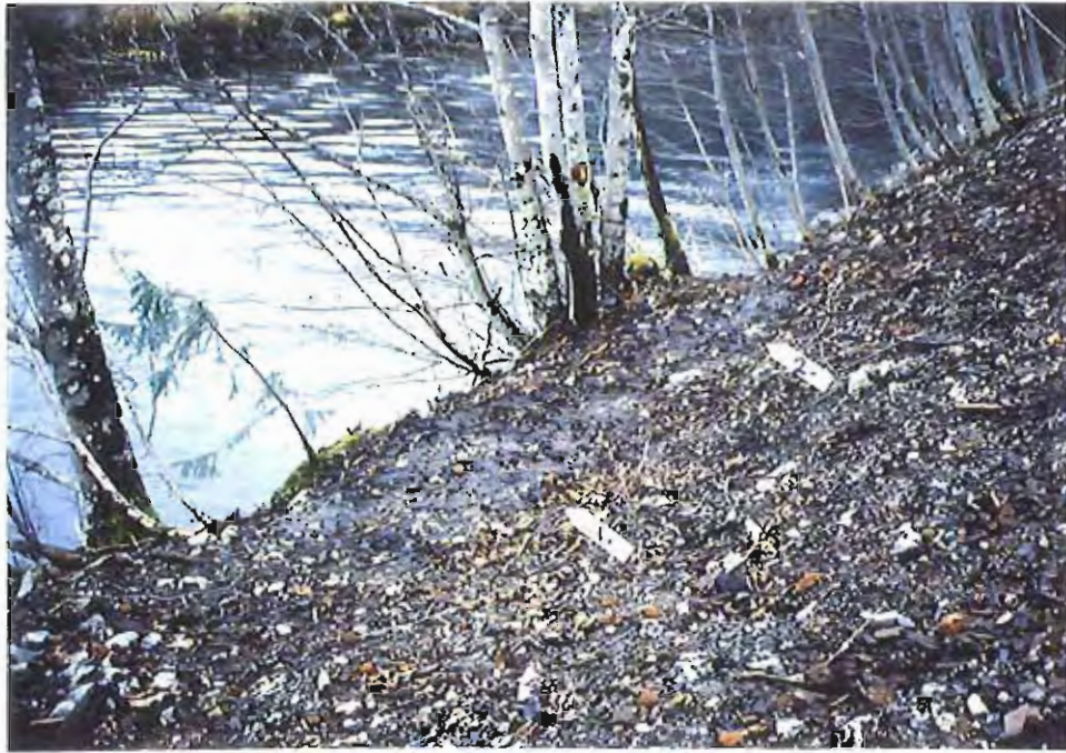
Photo #89 : Another 11/23/99 view of the two very small water seepages along the APC/Sitka landfill's embankment toe at about Sta. 3+60' to 3+80' (see next two photos).
