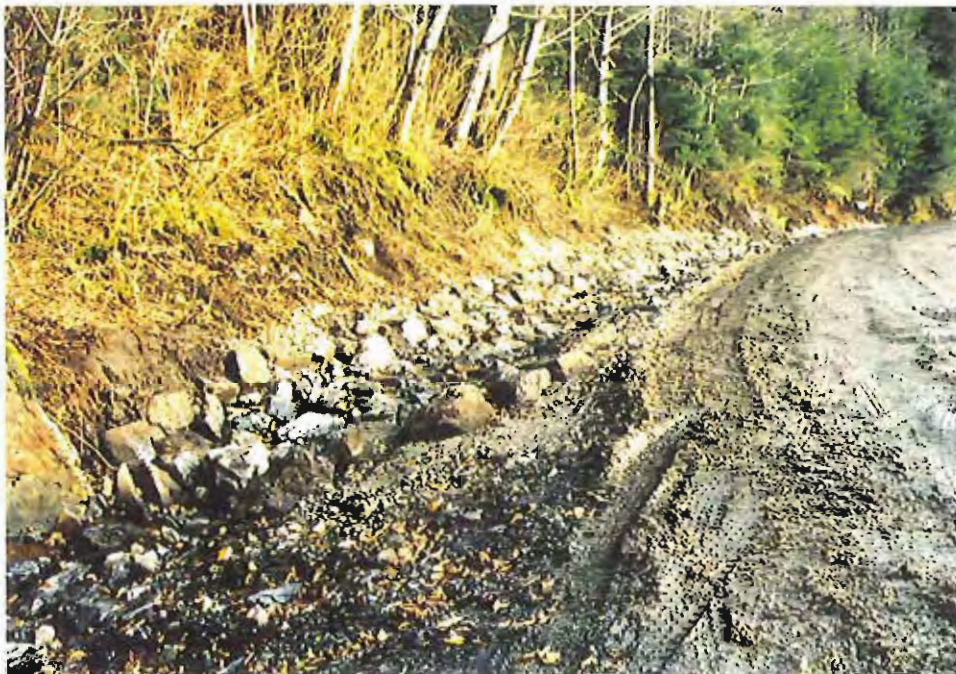
Photo #10: 11/11/99 view looking up the APC/Sitka landfill's upslope drainage ditch along Sawmill Creek Road taken from about Sta. 6+50', showing the large rock placed over the underlying 30-mil membrane liner to prevent surface water erosion.
