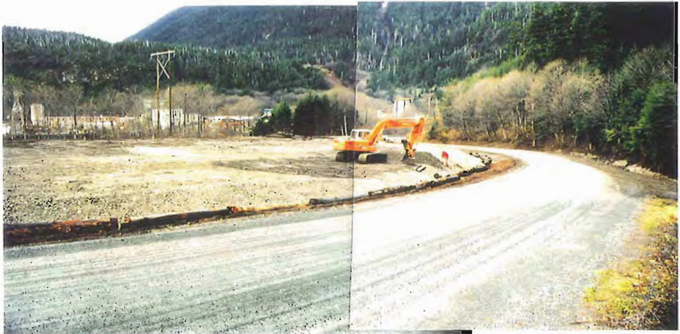
Photo #43: Looking northwest across the Sawmill Creek Road at the APC/Sitka landfill on 11/11/99, showing the spreading of crushed concrete over the top surface.
