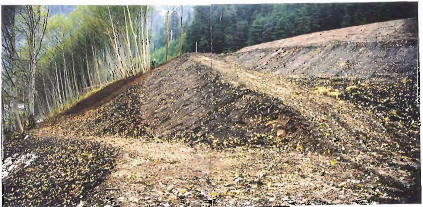
Photo #30: 10/20/99 view of the lower embankment of the APC/Sitka landfill, taken from about Sta. 2+00' and showing the completed placement of soil cover. The fresh-appearing soil along the far end of the embankment has just been hand-raked, to smooth out the soil that had been cast by the backhoe.
