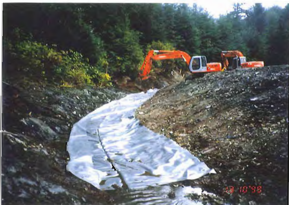
Photo #10: 10/13/99 view of the surface water drainage ditch along the upland side of the APC/Sitka landfill's northeastern area. Note that the left edge of its 30-mil liner is rolled back to allow the backhoe to dig a shallow trench where the liner's edge will be secured within the soil embankment (see next photo).
