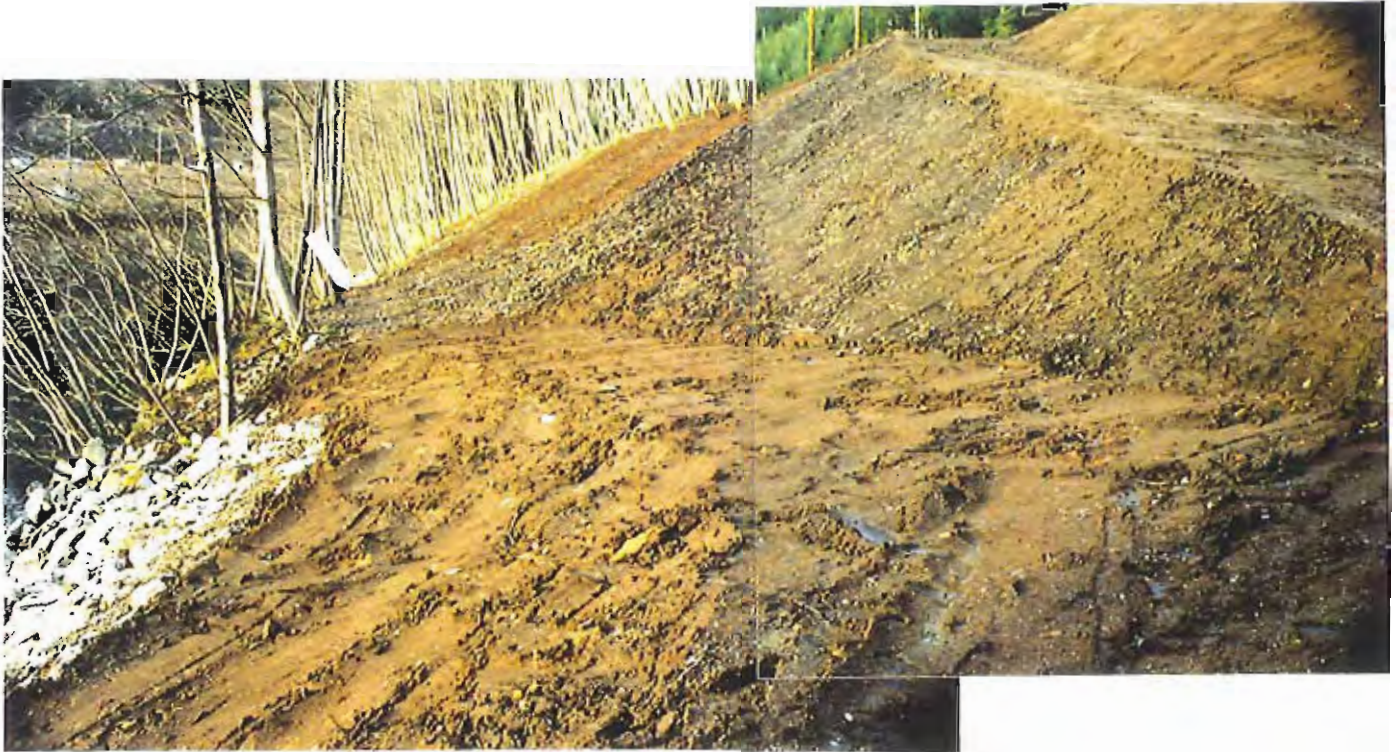
Photo #57: 11/11/99 view looking northwest from about Sta. 1+70' along the toe of the APC/Sitka landfill's embankment, showing the completed placement of the area's 6"-thick soil cover. Arrow points to the location of a very small water seep, refer to the photo below.
