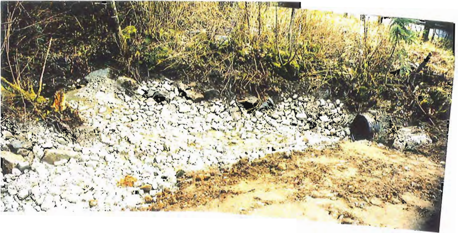
Photo #5: Looking down on the Sawmill Creek Road's culvert that goes through the APC/Sitka landfill's south end, showing the rock-lined creek which has a 30-mil membrane liner under the rock.
