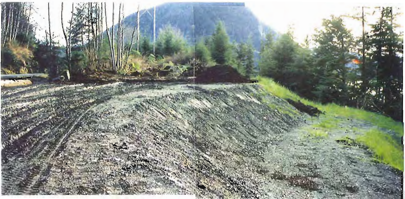
Photo #50: Closer view of the 6"-thick layer of surfacing soil being placed across the south end of the APC/Sitka landfill site on 11/11/99.
