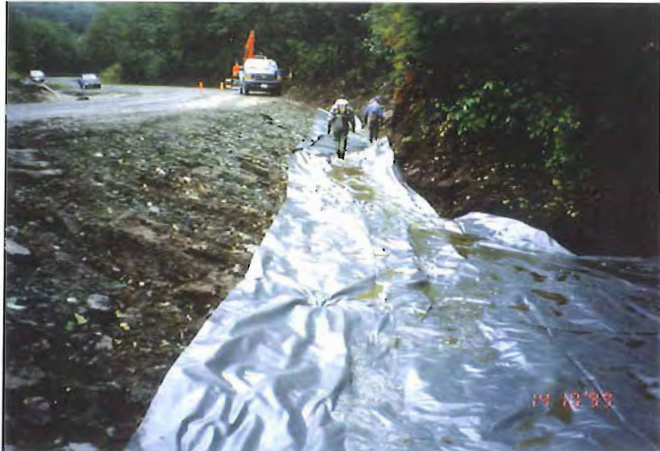
Photo #13: Laying of the 30-mil membrane liner along the Sawmill Creek Roadway's upland surface water drainage ditch on 10/14/99.
