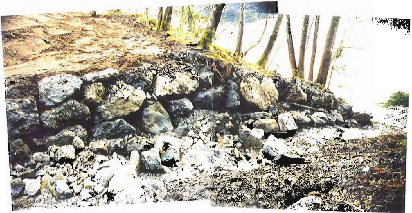
Photo #42: Closer 11/11/99 view near the end of the APC/Sitka landfill's northwestern surface water drainage ditch, showing the completed rockwork to protect against bank erosion.
