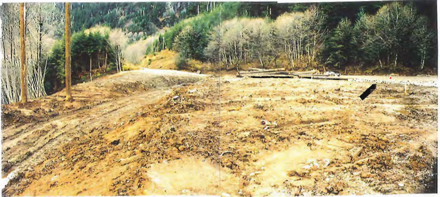
Photo #67: Looking north on 11/11/99 along the APC/Sitka landfill's top surface from about Sta. 3+50', showing the crushed-concrete surfacing fill beginning to be extended across the area (see arrow). Also shown in the far upper portion of the photo is the site's northwestern area, which still has to be covered with 18" of crushed rock and 6" of soil.
