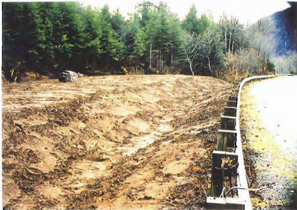
Photo #64: 11/11/99 view looking up the completed ditchline between the Sawmill Creek Road shoulder and the APC/Sitka landfill's northeastern disposal area, showing the area with its 6"-thick soil cover.
