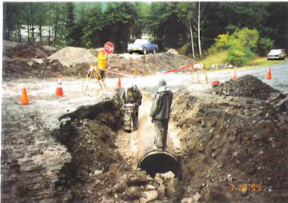
Photo #2: 10/7/99 view looking southwest at the inlet to the new 3'-dia. culvert being installed across the Sawmill Creek Road to drain the upslope surface water away from the APC/Sitka landfill deposits.
