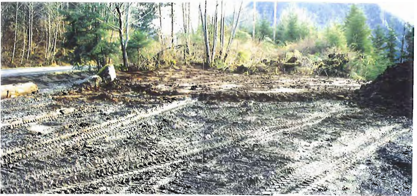
Photo #49: 11/11/99 view of the final 6"-thick surfacing layer of soil being placed along the south end of the APC/Sitka landfill.
