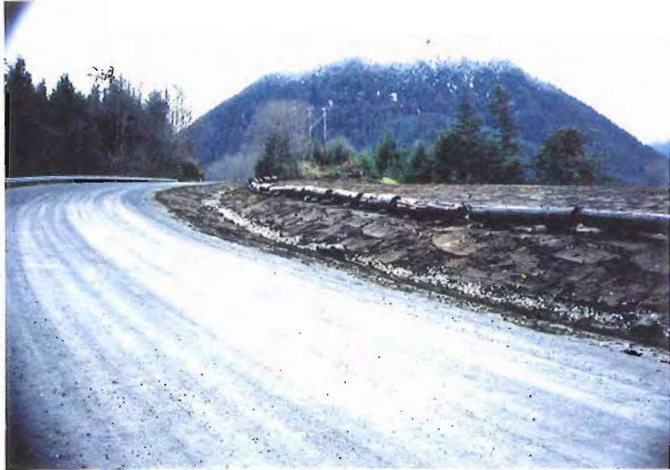
Photo #3: 11/23/99 view of the completed surface water drainage ditch along Sawmill Creek Road near the APC/Sitka landfill's southeastern end (compare with Photo #17).
