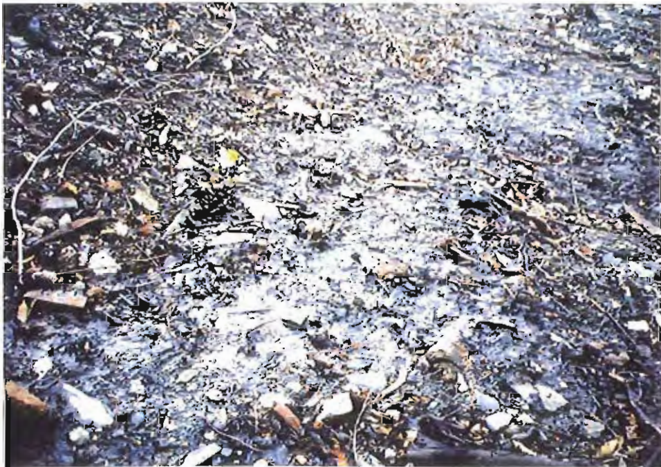
Photo #90 : Closer 11/23/99 view of the very small water seepage #1 along the APC/Sitka landfill's embankment toe at about Sta. 3+60' (see previous 2 photos for location).
