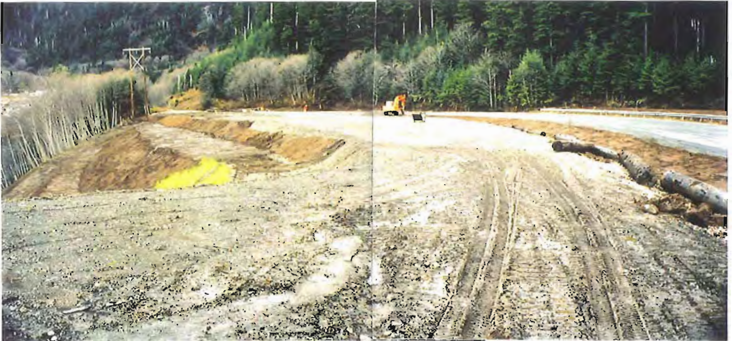
Photo #45: Looking northwest across the upper surface and embankment of the APC/Sitka landfill on 11/11/99. The crushed-concrete surfacing layer is completed throughout this area until just beyond the green hopper bin.
