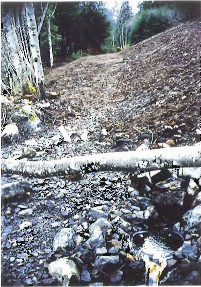
Photo #93: 11/23/99 view of a very small water seepage area (see arrow) just above the APC/Sitka landfill's water sampling site #1 which is in the lower right corner of the photo at about Sta. 5+50', refer to next photo.
