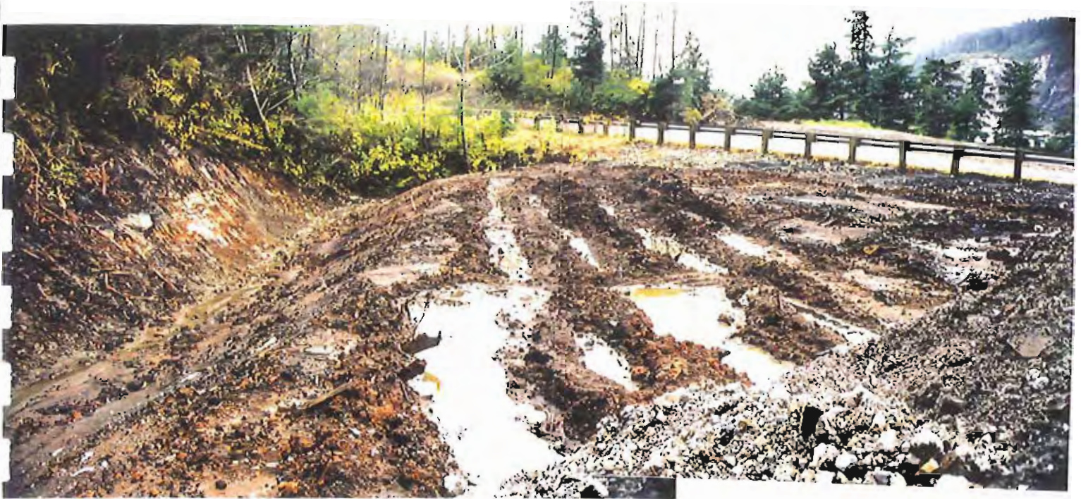
Photo #27: Looking south across the end of the APC/Sitka landfill's northeastern area on 10/20/99, showing the existing volcanic-ash soil cover's ability to provide a good seal for surface water drainage. A 1.5' layer of crushed rock will be placed across the surface, followed by a 4"-thick soil layer, and a 30-mil membrane liner will be placed in the ditch along the left side of the photo.
