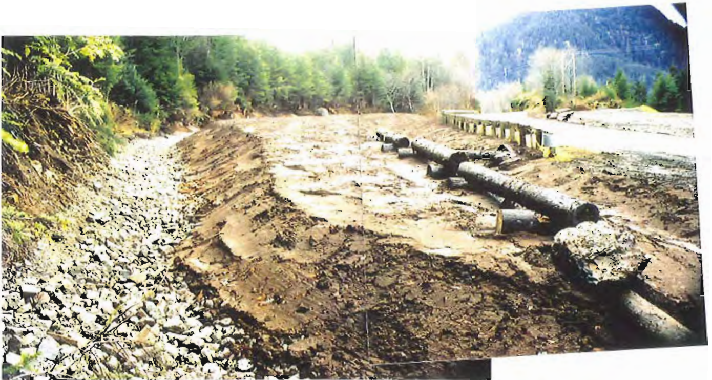
Photo #63: 11/11/99 view of the upslope surface water drainage ditchline around the APC/Sitka landfill's northeastern disposal area, showing the completed crushed-concrete rock now throughout the entire ditchline and the adjacent landfill's 6"-thick soil extending over the rock to the ditch bottom.
