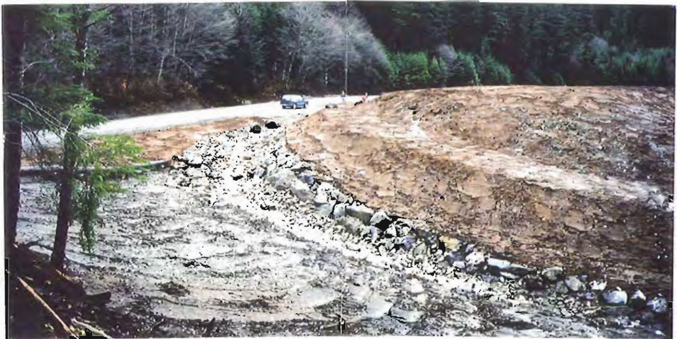
Photo #96: 11/23/99 view of the completed surface water drainage ditch around the APC/Sitka landfill's northwestern end, showing the gentle embankment slope along the roadside near the culverts, and the rock-lined ditch.
