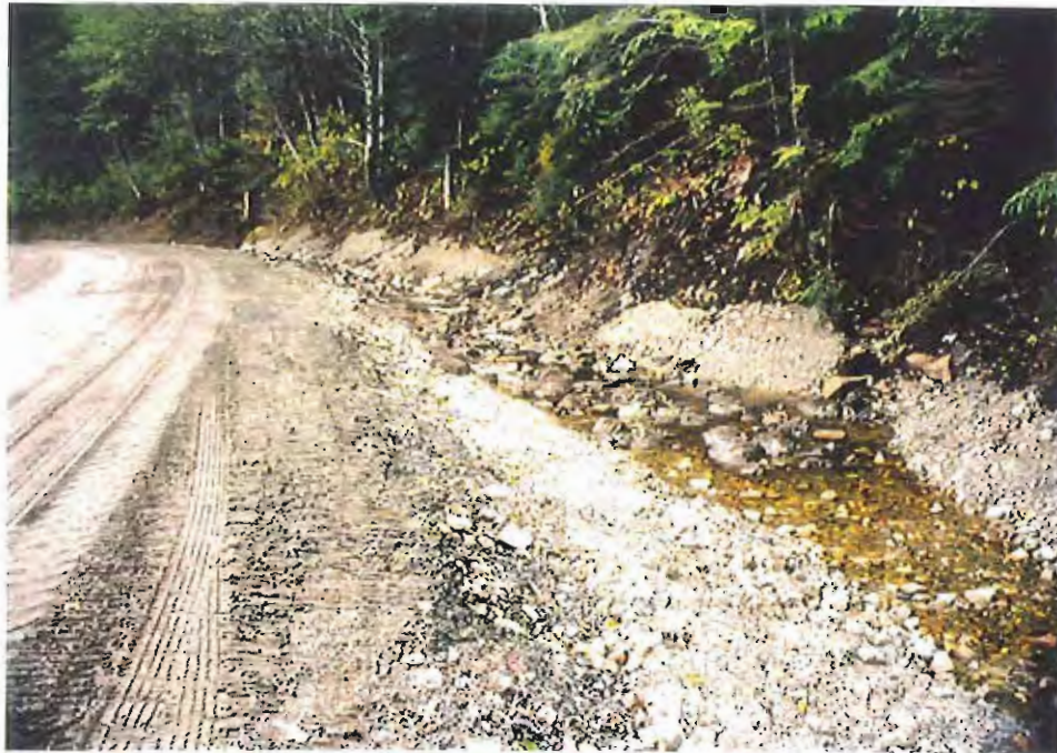
Photo #19: Looking down the nearly completed upland drainage ditch along the Sawmill Creek Road from about Sta. 3+50', showing the substantial water flowing in the ditch, 10/20/99.
