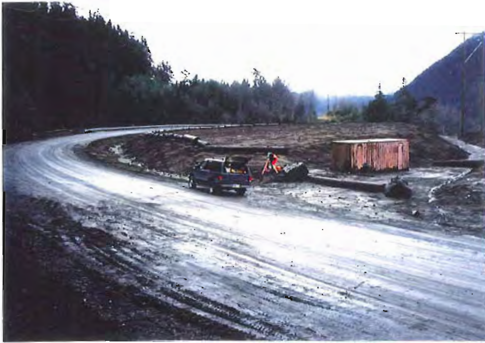
Photo #1: 11/23/99 view looking southeast across the main portion of the APC/Sitka landfill site, showing the Sawmill Creek Road and the completed downslope ditchline.
