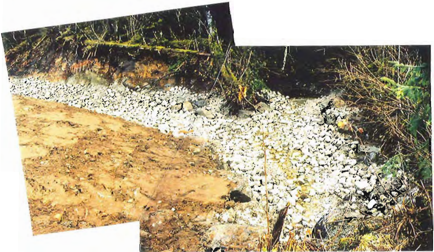
Photo #66: 11/11/99 view looking across the small creek entering the south-end culvert at the APC/Sitka landfill site, showing the crushed-concrete surfacing that completely covers the 30-mil liner that underlies the entire rocked area. The upslope drainage ditchline extending to the right is lined with four 6-mil plastic layers, followed by a 6"-thick layer of crushed concrete.
