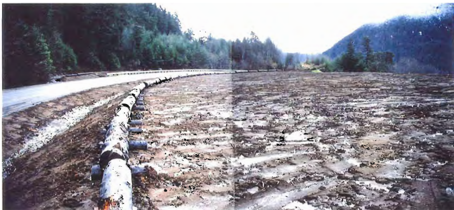
Photo #80: 11/23/99 view looking southeast along the new barrier logs separating the completed ditchline by the roadway from the main top surface of the APC/Sitka landfill site.
