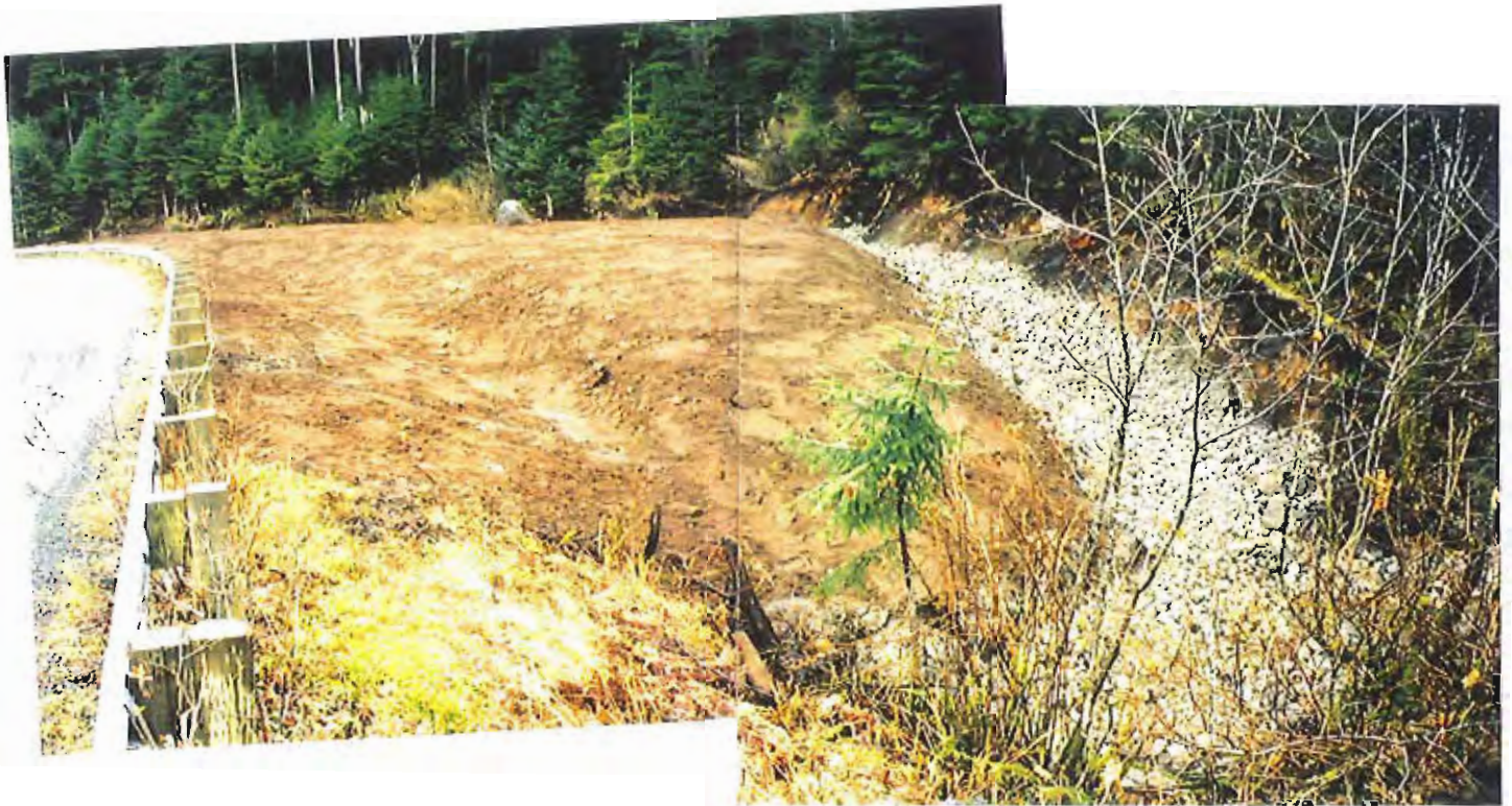
Photo #65: 11/11/99 view looking across the APC/Sitka landfill's northeastern area, showing its completed upslope ditchline and the 6"-thick covering of soil throughout the area which extends to the roadway's edge.
