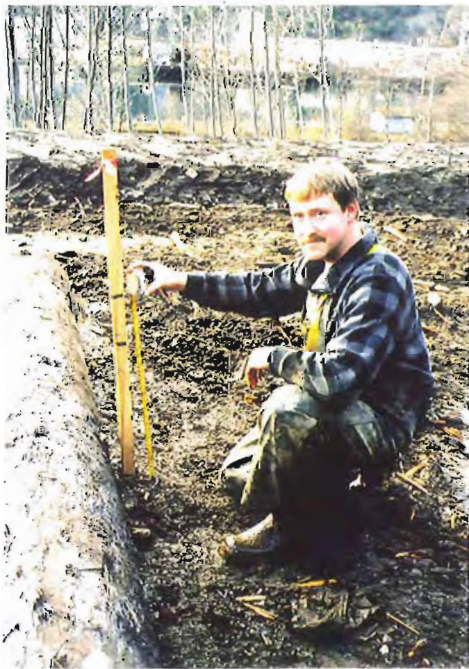
Photo #48: Close-up view of the survey stakes being marked to assure that the crushed-concrete fill is 18" thick throughout, followed by a 6"-thick layer of soil.
