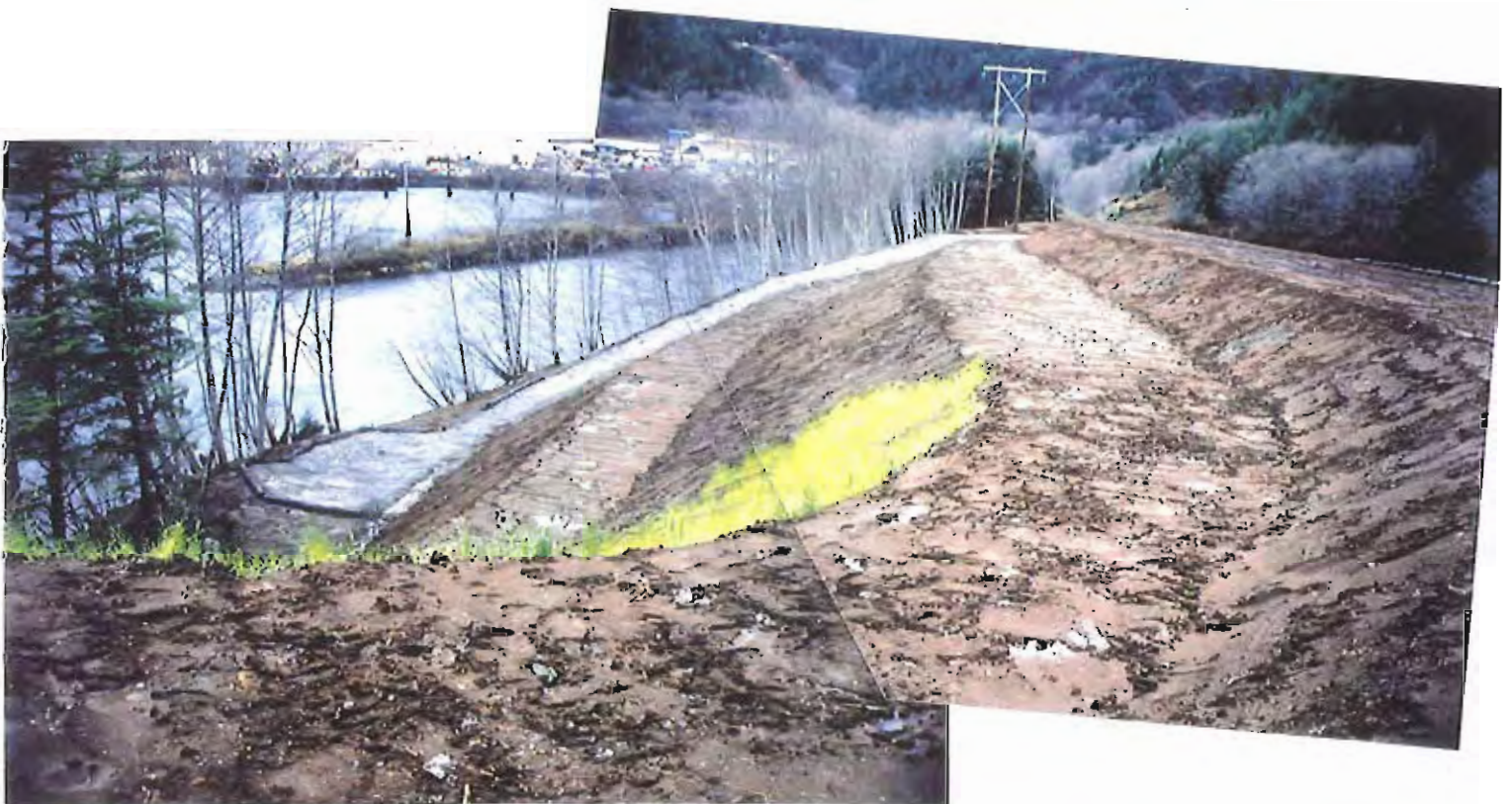
Photo #84: 11/23/99 view looking across the terraced outer embankment of the APC/Sitka landfill site, showing the final 6"-thick soil layer in place and the access road to the bottom of the embankment now surfaced with crushed concrete fill and lined with creosoted logs.
