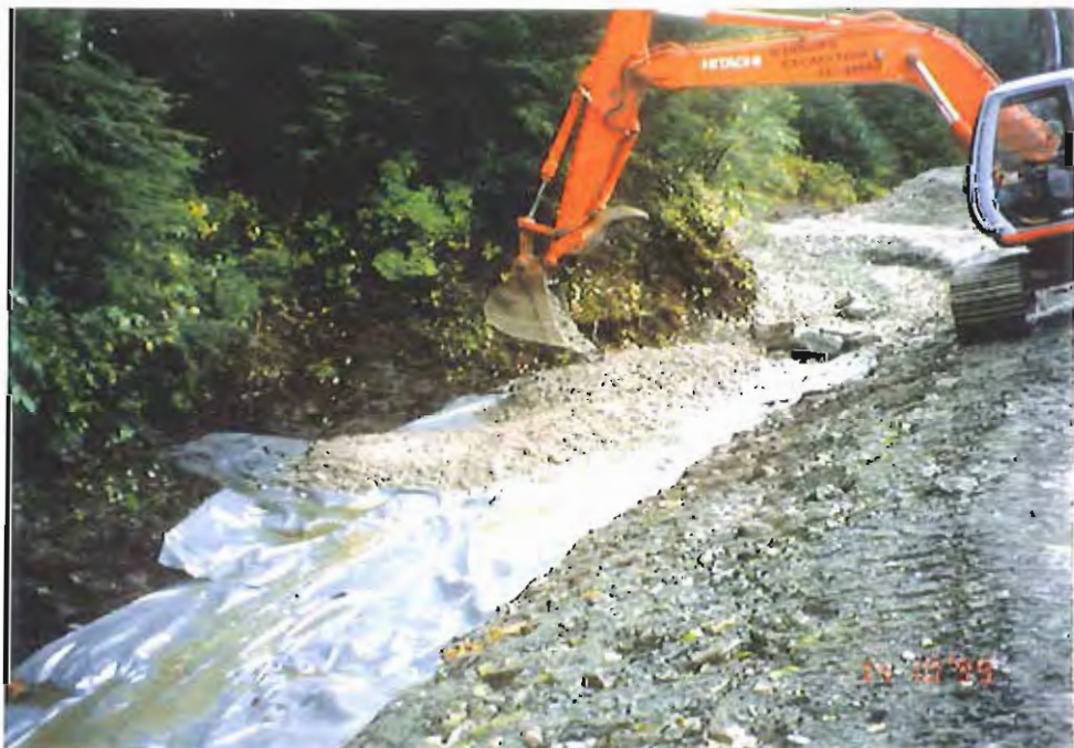
Photo #14: Continued placement of the 6"-layer of crushed concrete over the 30-mil membrane at about Sta. 3+50' in the APC/Sitka Landfill's ditch, along the upland side of Sawmill Creek Road. Note the extension of liner to catch the small stream coming in from the left side of the photo.
