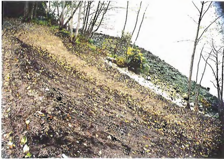
Photo #31: 10/20/99 view looking down the APC/Sitka landfill embankment from about Sta. 3+00', showing the complete covering of soil that extended to the stabilization rock along the tidelands.
